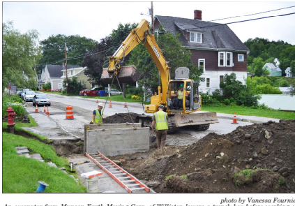
An excavator from Munson Earth Moving Corp. of Williston lowers a trench box before working on installing a new fire hydrant Friday. This was the last of the main waterline installations for Church Street, Maple Street, Slaggy Hill and Vermont Avenue. Spot paving is scheduled to begin this week.
