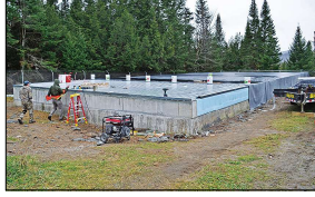
Construction continues on the town reservoir on Bigdollar Hill in Hardwick. Last week, site prep superintendent Dana Spotts of Spotts Construction, Inc. led by and Town Manager Shaun Fiedler. The work will be done at the facility, completed, which began the end of September, is scheduled to be constructed by the end of December.
