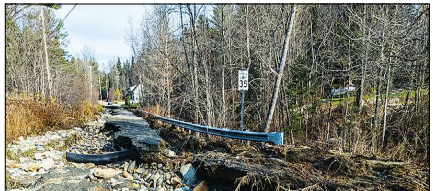
photos by Enoch McGraw Broad Road at North Wolcott Road in the aftermath of the Halloween storm. The road washed out and debris is everywhere.
