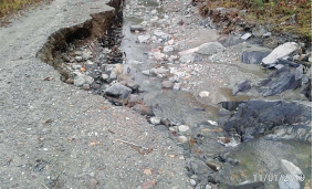
courtesy photo from Bruce Urie Town Line Road in Craftsbury became a tangle of debris, mud, and water by early Friday morning, with wash-ups more than six feet deep. Quick responses by the road crew, Dwight Detton, and others made it possible to restore the road into a one-lane passage by Friday afternoon.
