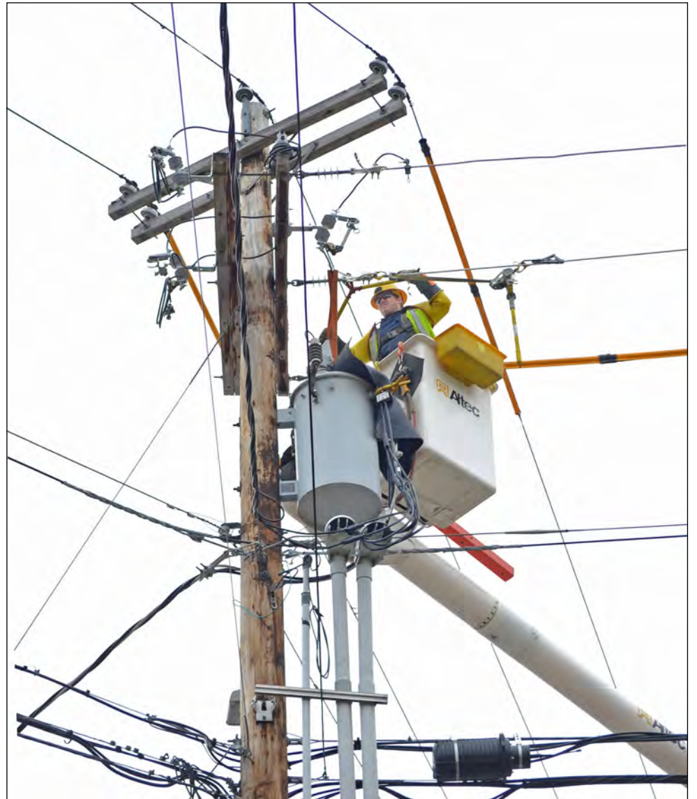
photo by Vanessa Fournier Hardwick 1st class lineman Tyler Kirkpatrick dead ends a replacement wire to a pole on North Main Street in Hardwick last week as part of an upgrade to that section of the system.
