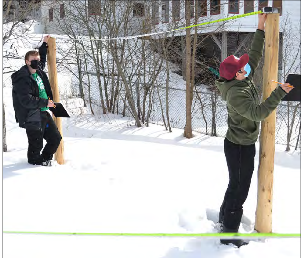
photo by Vanessa Fournier Cabot middle school students Ethan Garrison (left) and Ben Monaco (right) take measurements and work on their design for a covering for an outdoor classroom during a Science and Social Studies project block. The outdoor structure will be located between the Cabot Performing Arts Center and the school library.
