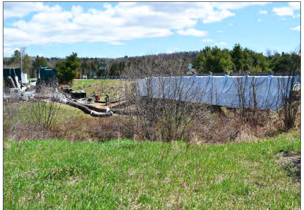
photo by Vanessa Fournier Construction on the Vt. Rte. 16 bridge #1 as seen from Route 15 in Hardwick.
