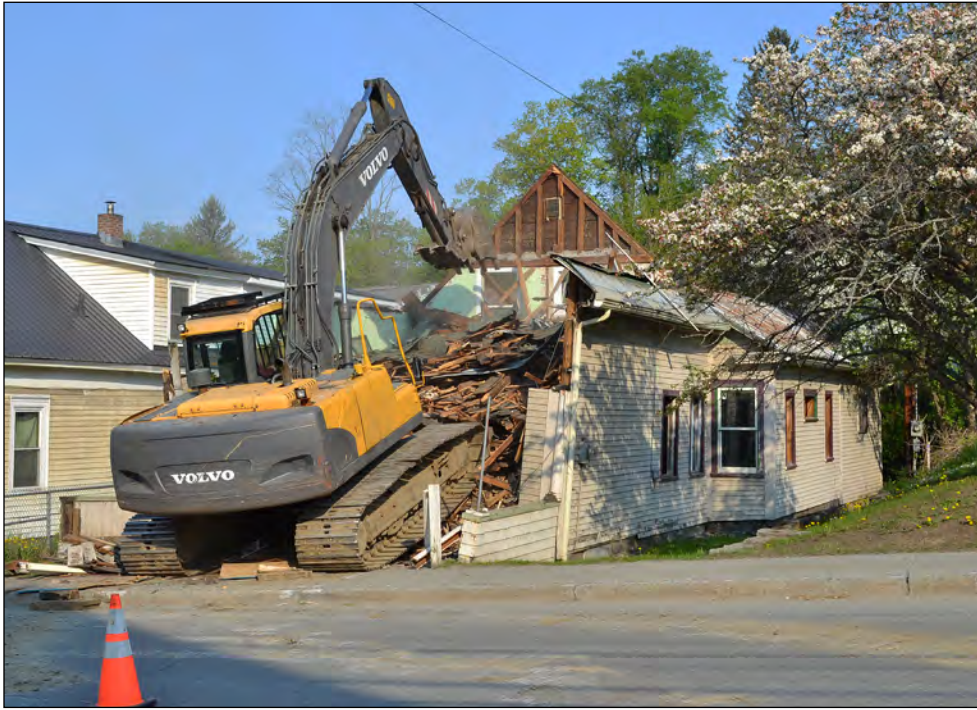
photo by Vanessa Fournier Raymond Lefevre of All Metals Recycling runs an excavator on May 19 as he tears down the former Senior Center building located on North Main Street beside the Jeudevine Library.
