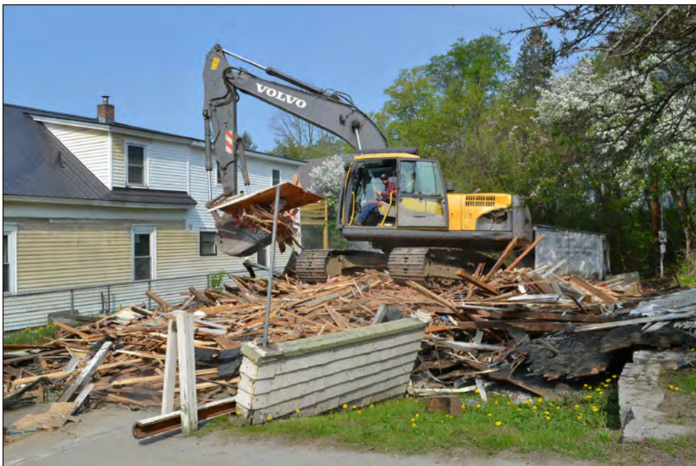
photo by Vanessa Fournier One and a half hours after the start of demolition work on the former Senior Center the building was down.
