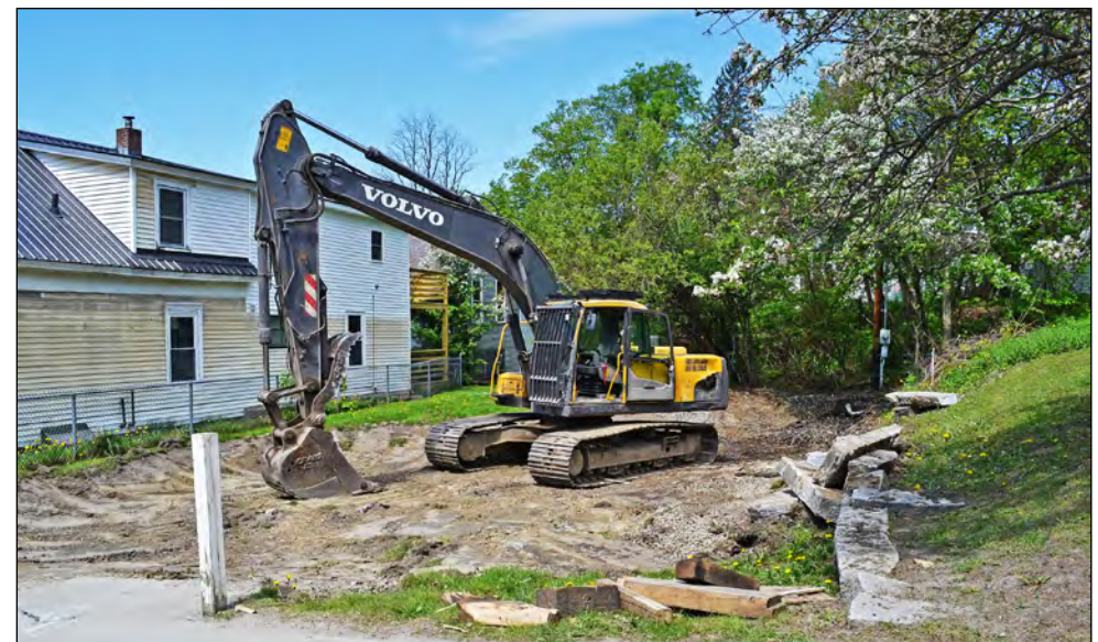
photo by Vanessa Fournier The day following the demolition of the former Senior Center the lot was empty.
