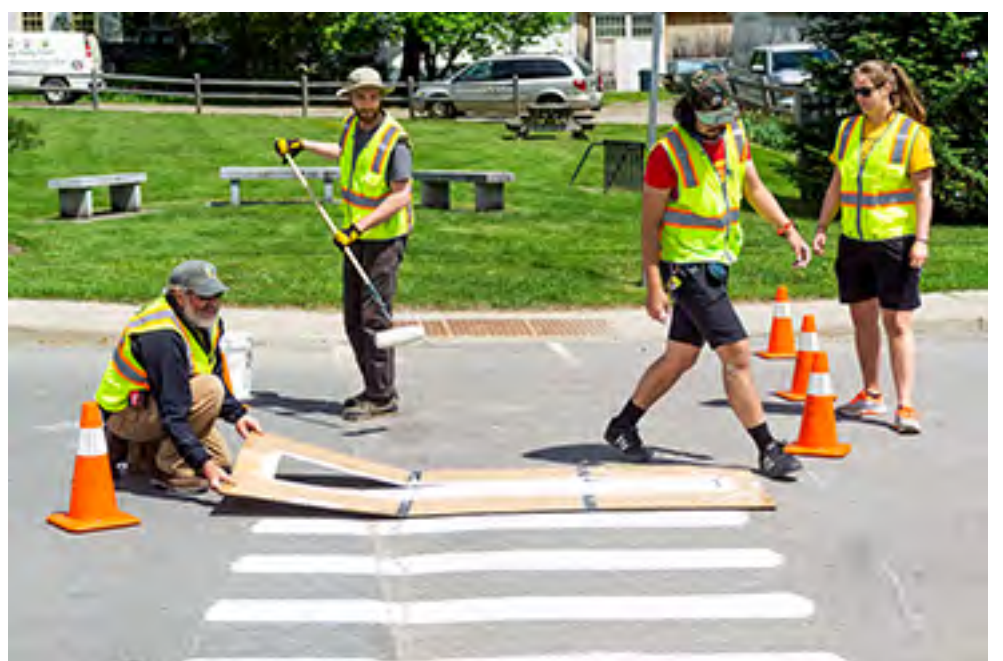
photo by Doug McClure Local Motion workers Keith Wight, Jonathon Weber, Tanawat Luerkr-u-suke and Sarah Illingworth work to install a temporary crosswalk at the intersection by the Willeys Store. The town, along with Local Motion, created a temporary mockup of proposed changes to the traffic flow and pedestrian access for Memorial Day weekend to see what impact those might have.
