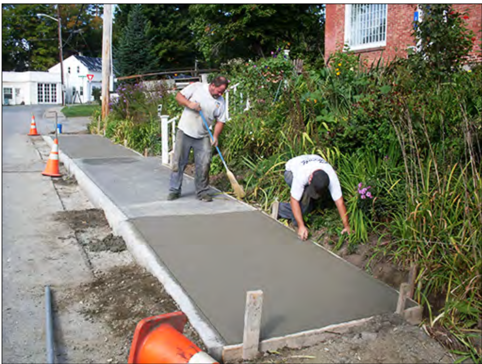
photo by Hal Gray Jeff Perry and his son, Jaden, of Brian Perry & Sons Construction, Inc. "finishing" (i.e., edging, sweeping, etc.) a section of the new Greensboro East Street sidewalk on September 17.
