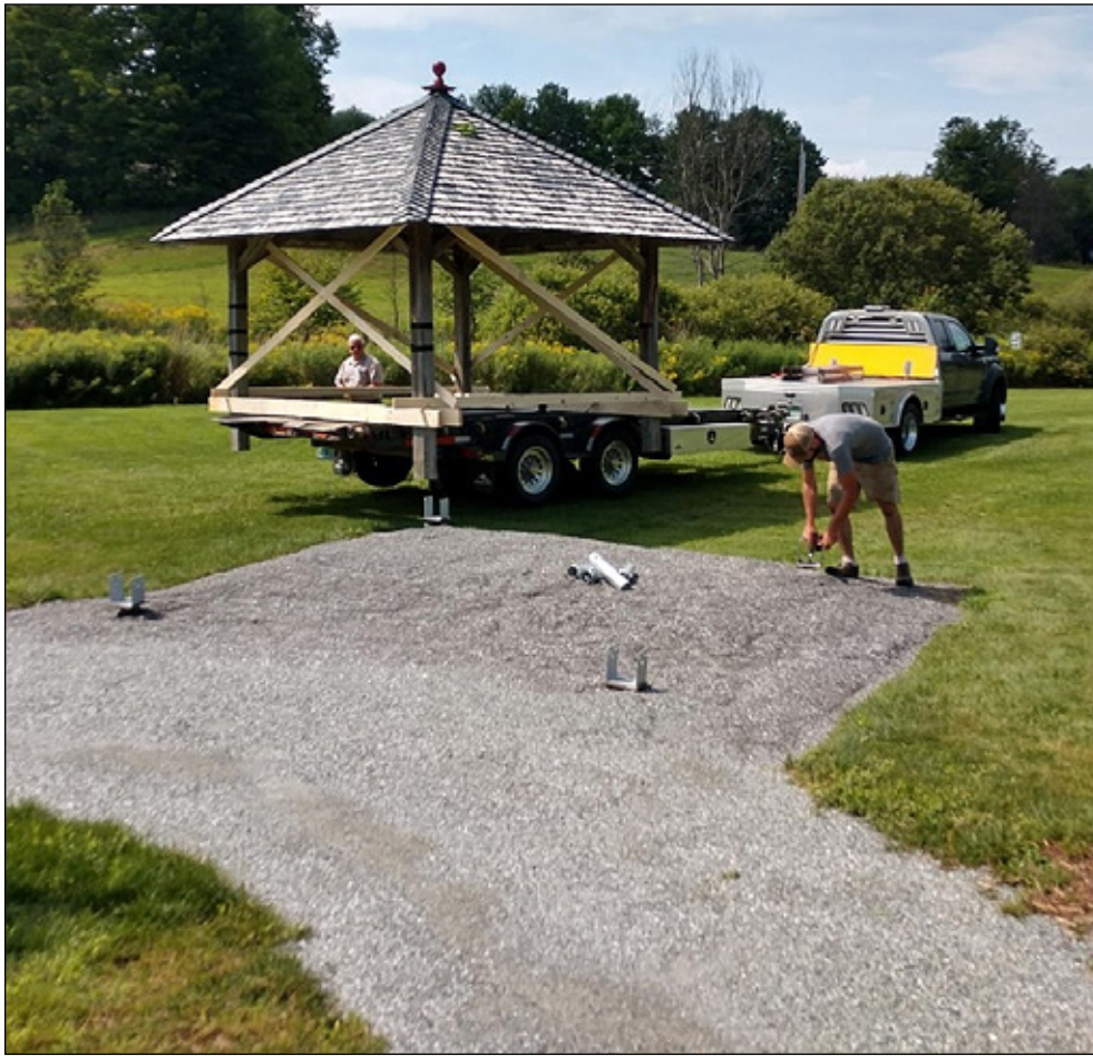
courtesy photo Glen Burkholder of Town & Country Sheds maneuvers a donated pavilion into place at the Craftsbury Community Care Center as Cody Thompson of C.T. Stoneworks fine-tunes the brackets.
