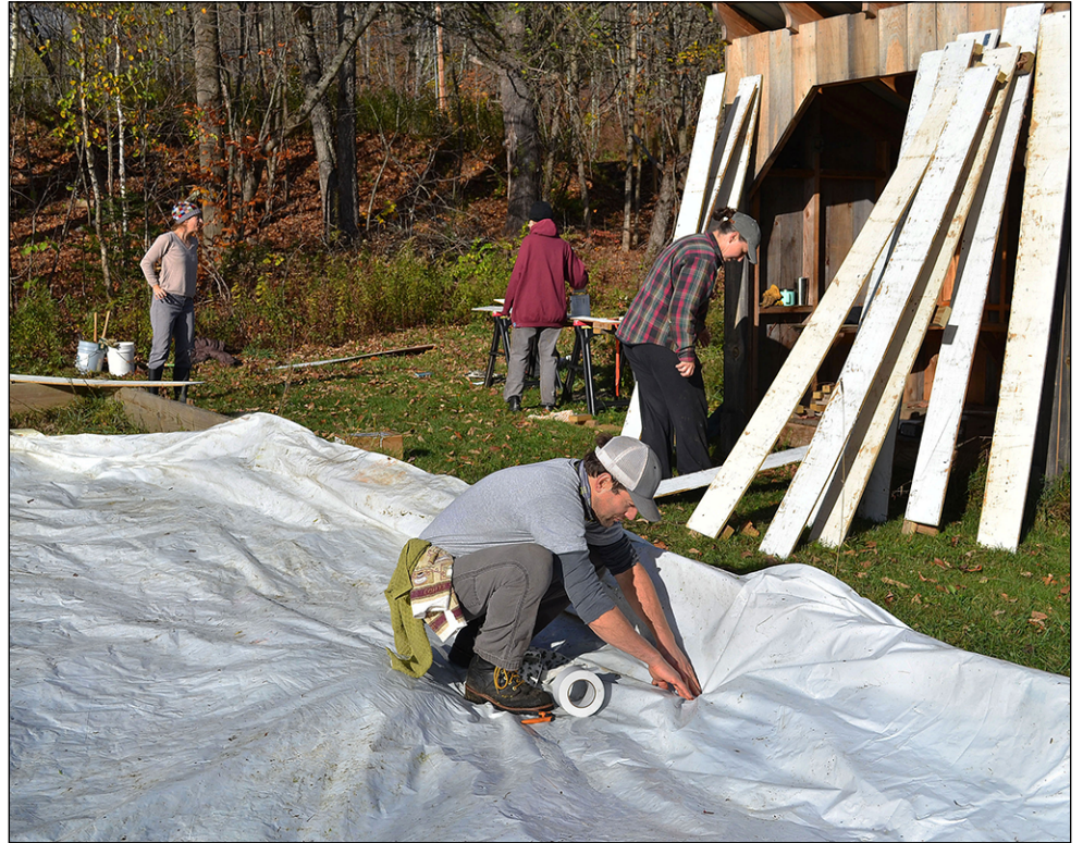
photo by Vanessa Fournier Saturday was the Woodbury Community Ice Rink workday. Volunteer Alex Peltz (front) makes repairs to the liner as Cindy Gordon, Laura Murphy and Elizabeth Stratton (in back from left) work on and paint the side boards. Six volunteers spruced up the 32 x 64-foot rink, getting it ready for its 6th season. Not pictured are Michael Gray and Steve Freihofner.
