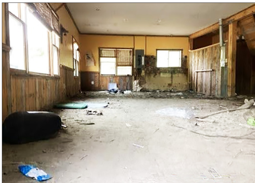
The interior of the home at 2832 Craftsbury Road in Hardwick following July 2023 flooding that swelled a stream beyond its banks, filling the home with over four feet of muddy water, leaving it uninhabitable.
