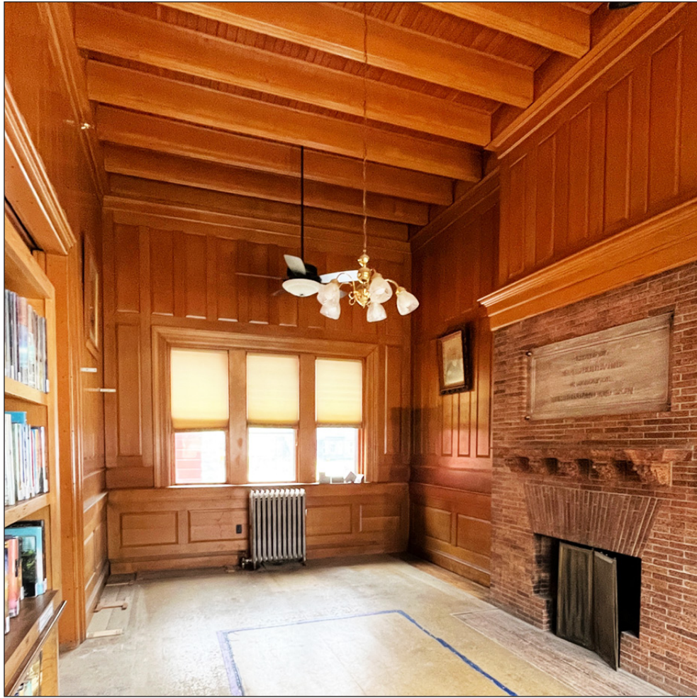
The library Children's Room, emptied of books and furniture, with carpeting removed for the floors to be refinished, will contain some of the adult collection and reading areas.
