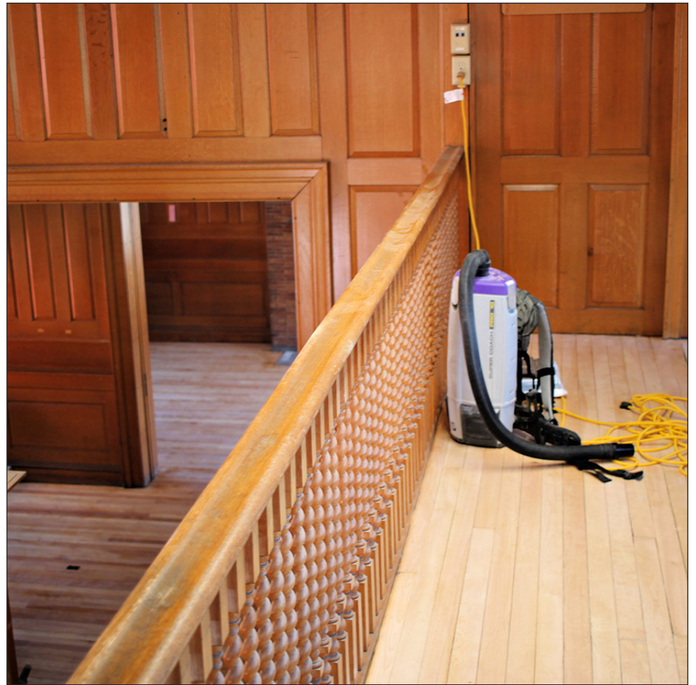
The upstairs balcony area of the original library has been cleared out to prepare for its floors to be refinished as the library's new addition nears completion.
