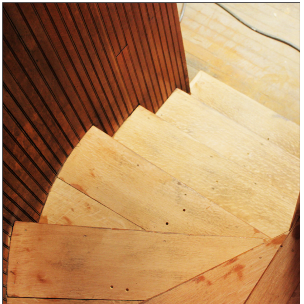
The original library's circular stairs leading to the upstairs balcony area have been sanded to prepare for their refinishing.
