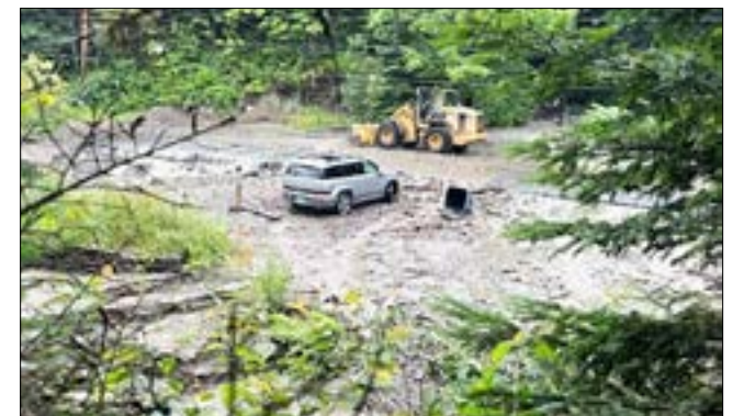
Craftsbury Road in Hardwick flooded for a second time on July 9, 2024. The equipment from the demolition was still on site when the second flood occurred. courtesy photo
