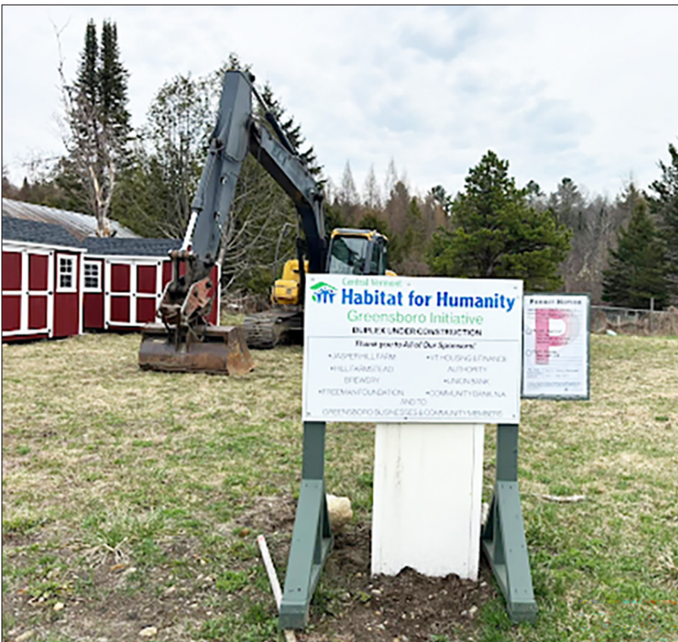
An excavator at 1119 Main Street in Greensboro Bend stands ready for work on the foundation of a new Habitat for Humanity duplex home. It began excavating for the building's slab on grade and frost walls, Monday, April 28. social media photo
