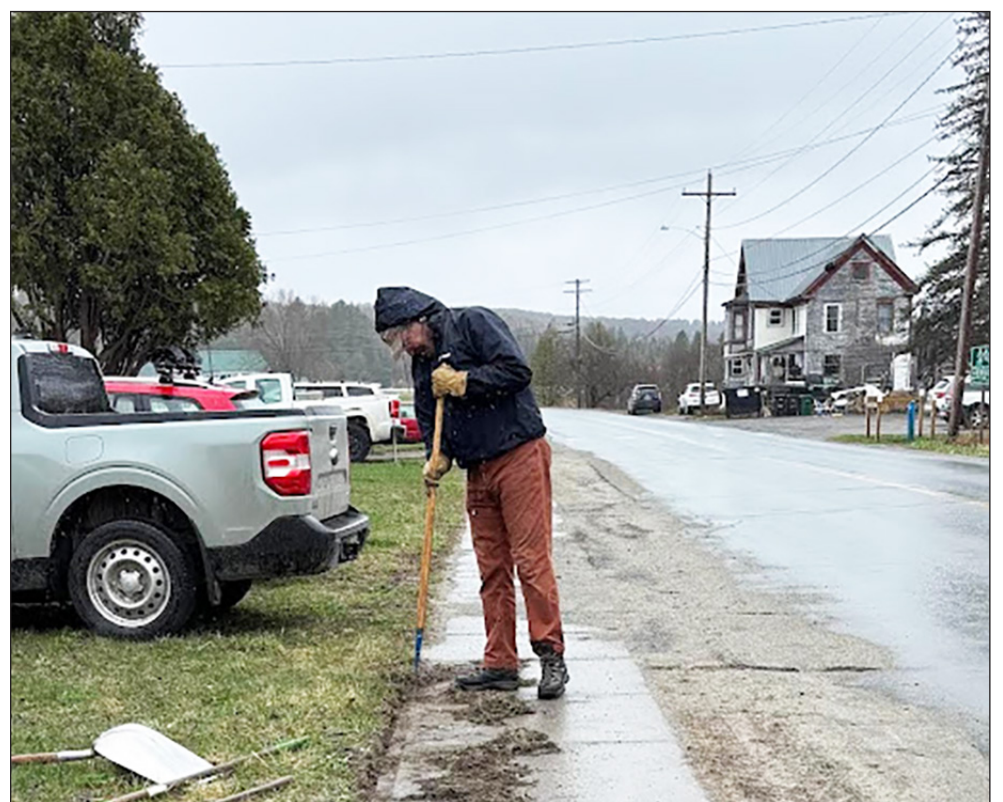
Rick Ely carefully edges the sidewalk at 1119 Main Street in Greensboro Bend, April 26, to assure accurate measurements for the foundation setback of a new duplex home planned by the Greensboro Initiative of Central Vermont Habitat for Humanity. photo by Jennifer Bayles
