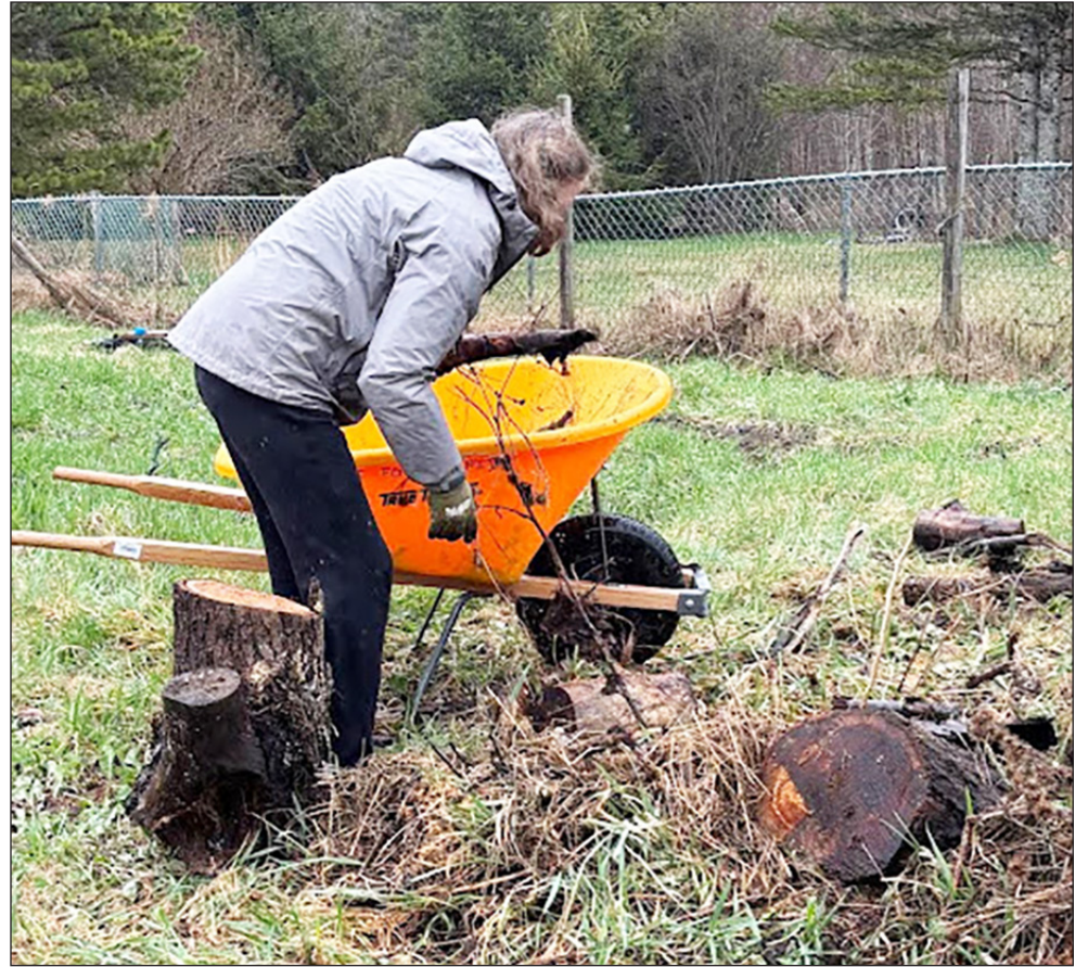
Kathy Hansen loads sawn logs into a wheelbarrow, April 26, at the site of a new Habitat for Humanity home in Greensboro Bend. They were given to a neighbor next door for firewood. photo by Jennifer Bayles
