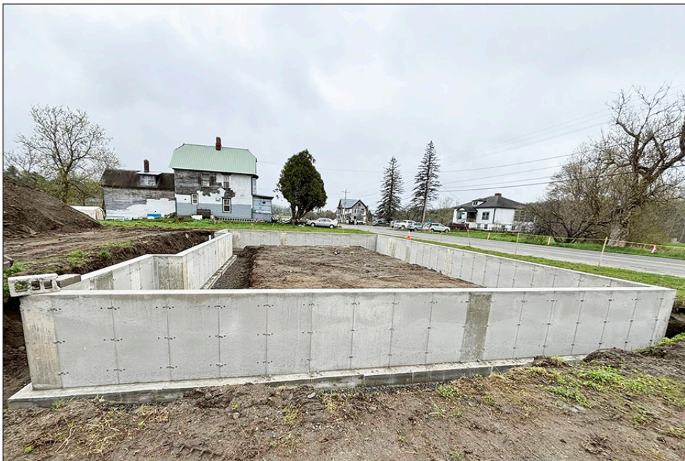
A poured concrete foundation, May 8, at 1119 Main Street in Greensboro Bend is the first evidence of the two-family home being constructed on the site by the Habitat for Humanity Greensboro Initiative.
