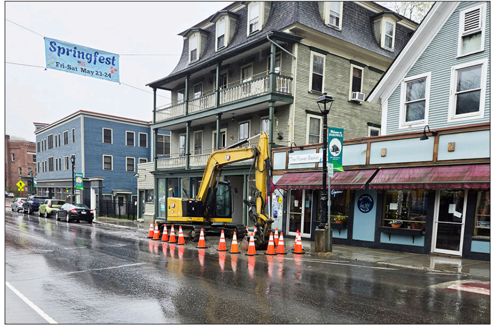
Cones around an excavator from Thursday through Saturday last week were the only daytime evidence of nighttime work on a South Main Street water leak in front of the Flower Basket. The repair was the subject of a series of alerts sent to town residents who had signed up for the town’s new alert notification system, which can be used to send notification to residents about water and wastewater issues, emergency response and other town business.
