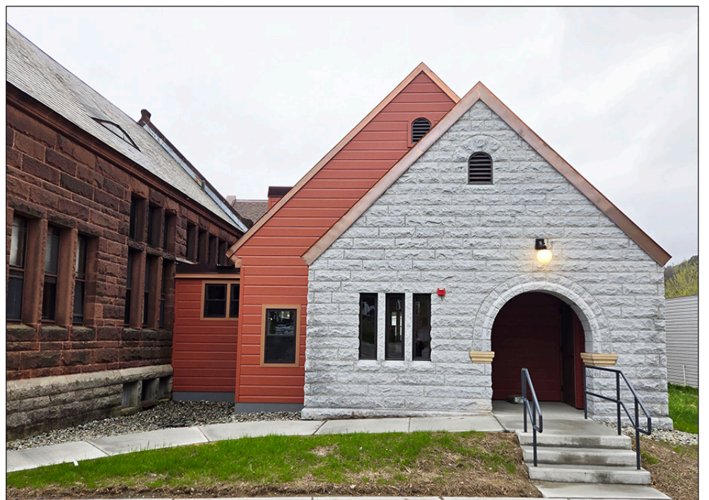
An exterior light came on above the new entrance to Hardwick’s Jeudevine Library for the first time last week, as the library addition nears completion, with a hoped for soft opening Memorial Day weekend, according to Librarian Diane Grenkow.
