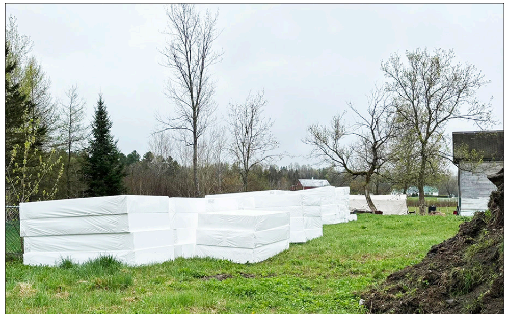
Foam Panels at the site of the Habitat for Humanity Greensboro Initiative, May 8, await volunteers at a work day scheduled for Monday, May 12. Six to eight volunteers were being recruited for dirty and messy work to help move, cut and adhere foam panels to the cement foundation walls.
