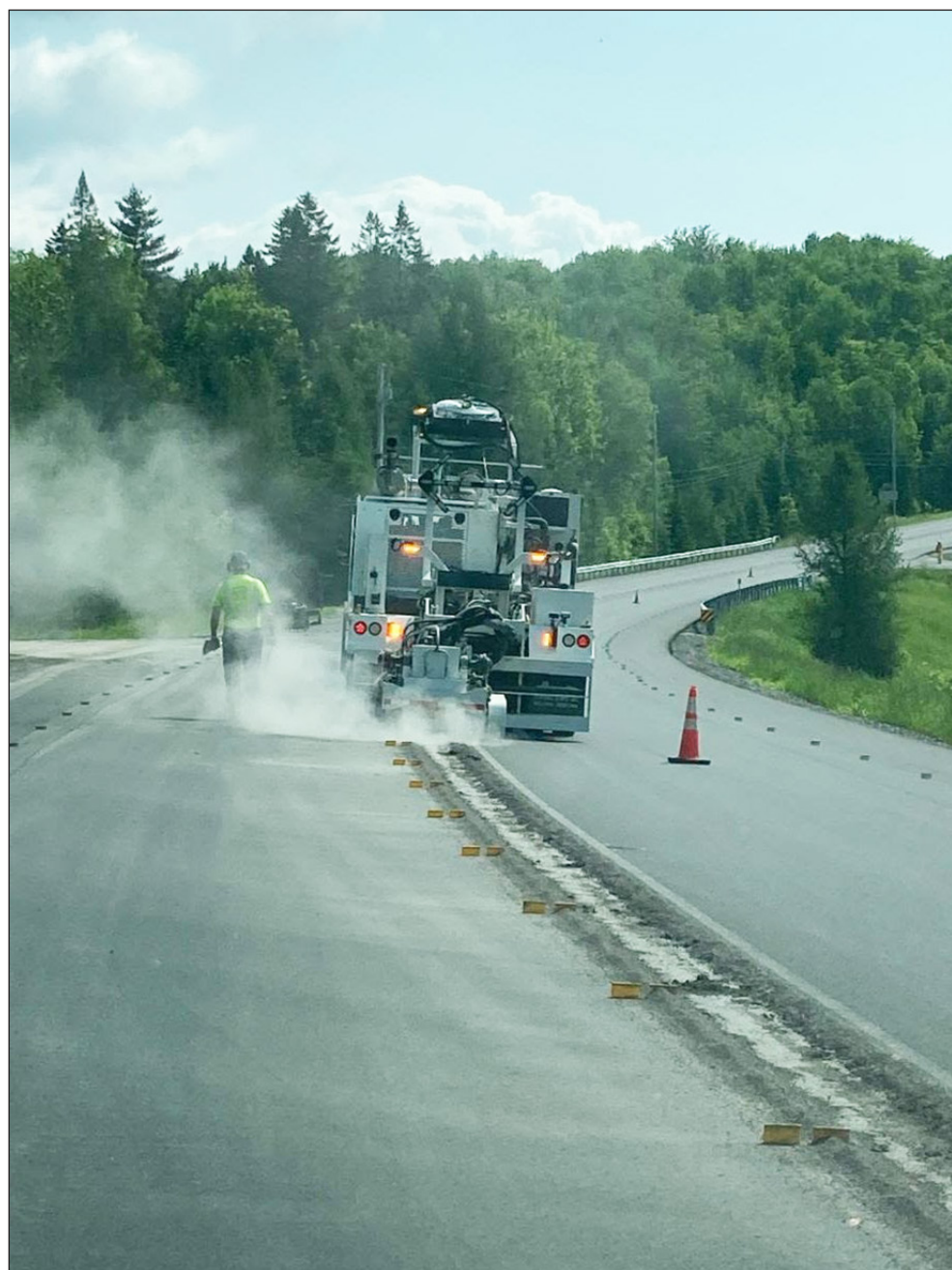
A VTrans construction crew installs center line rumble strips during the resurfacing of U.S. Rte. 2 photo courtesy VTrans
