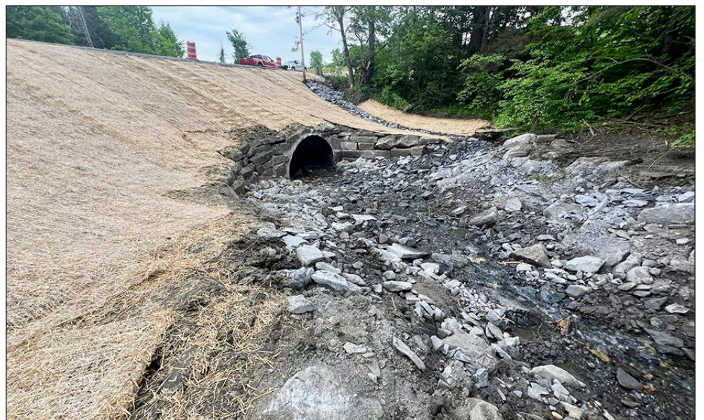
Work on a new culvert under Menard Road had been completed last week, except for the addition of guardrails.
