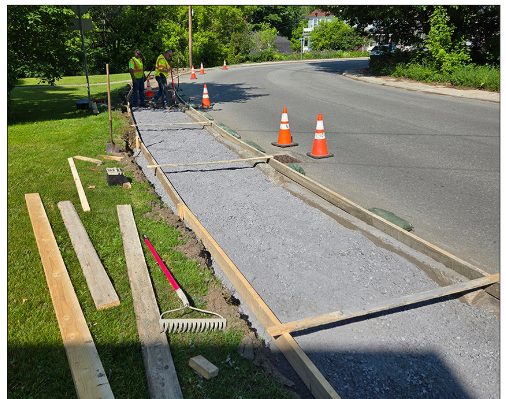
Hardwick Road Crew members Barry McLaren (left) and Perley Allen set forms for new sidewalks in front of the Maple Street Apartments, Monday, June 16. They plan to continue down that side of Church Street and around the corner at the Memorial Building onto N. Main St. this summer.
