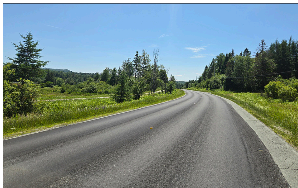
New patches on the Vt. Route 16 pavement through Greensboro Bend have not yet had new lane marking applied, Friday, June 27.
