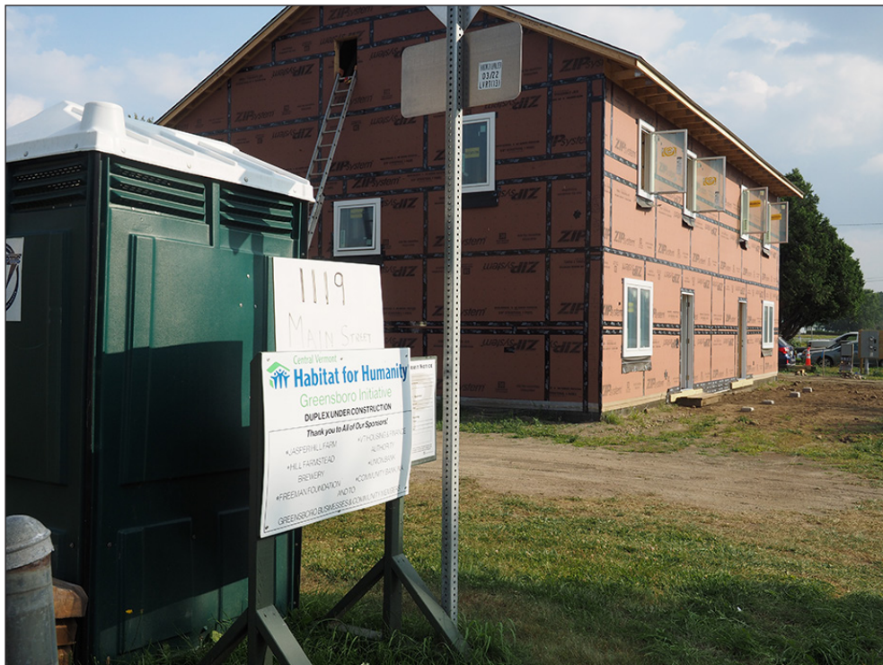
A new Habitat for Humanity duplex home is being built at 1119 Main St.
