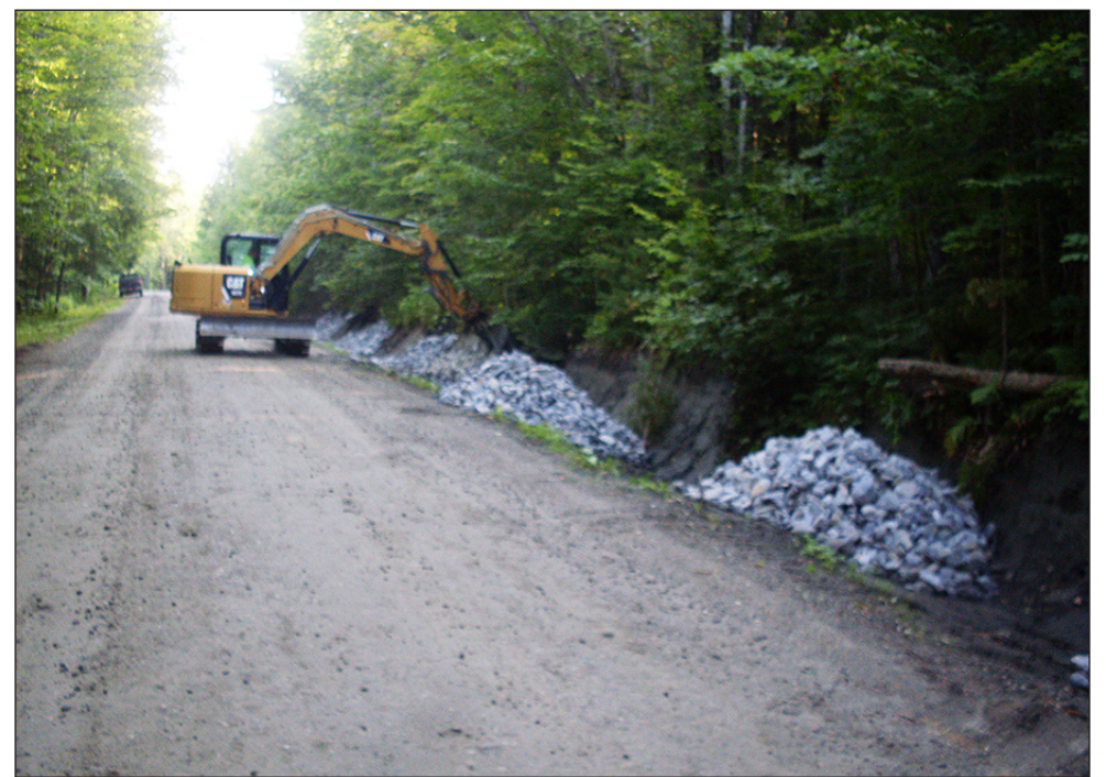
Piles of rock await distribution in the ditch by the excavator as a means of rainwater management. along Greensboro's Lakeview Road. August 11. photo by Hal Gray
