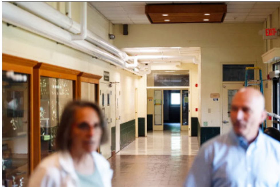
A once-temporary but now permanent fix to the heating system are seen in pipes suspended along the hallways of Woodstock Union High School.
