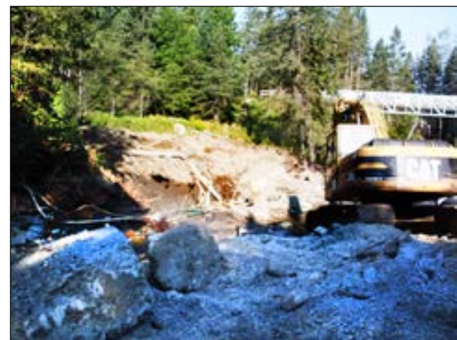
Construction continues on a new Orton Road bridge in Greensboro, August 11, as the road joins the Stannard Mountain Road, just east of the Lamoille Valley Rail Trail on the upper right.
