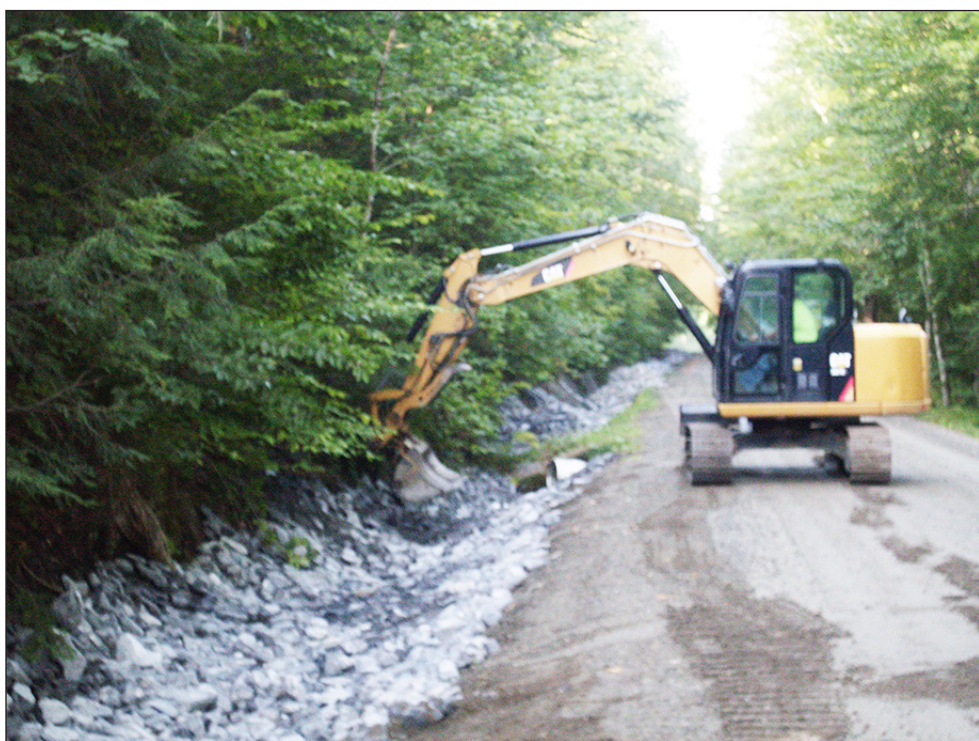
An excavator lines a Greensboro Lakeview Road ditch with rock, August 11, as a means of rainwater management. photo by Hal Gray
