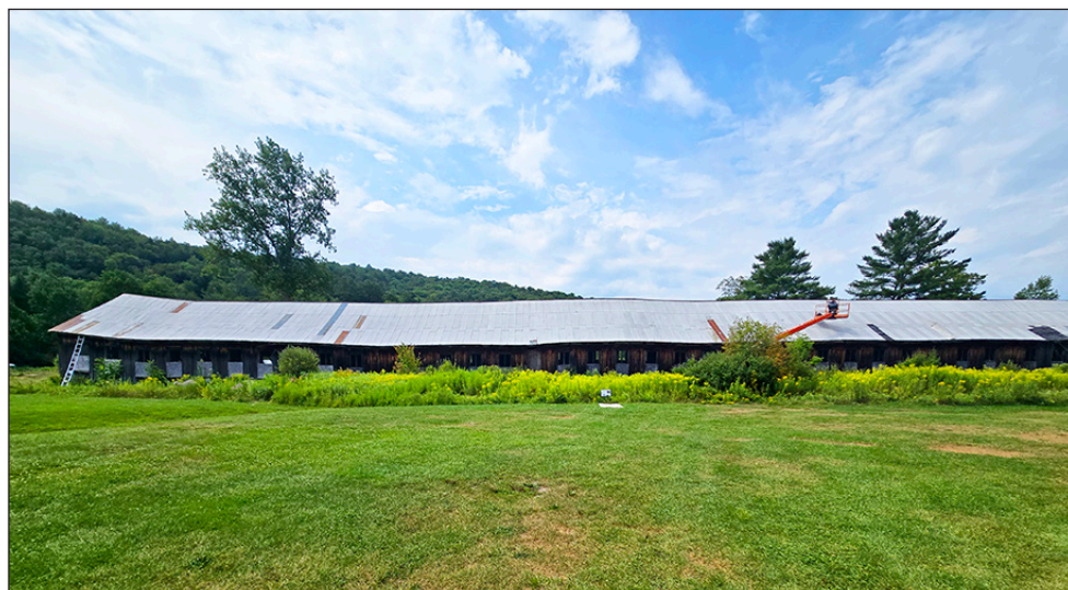
Junior Cisneros and his crew from JR Quality Construction work to repair and replace sheet metal roofing on Hardwick's Atkins Field granite shed.
