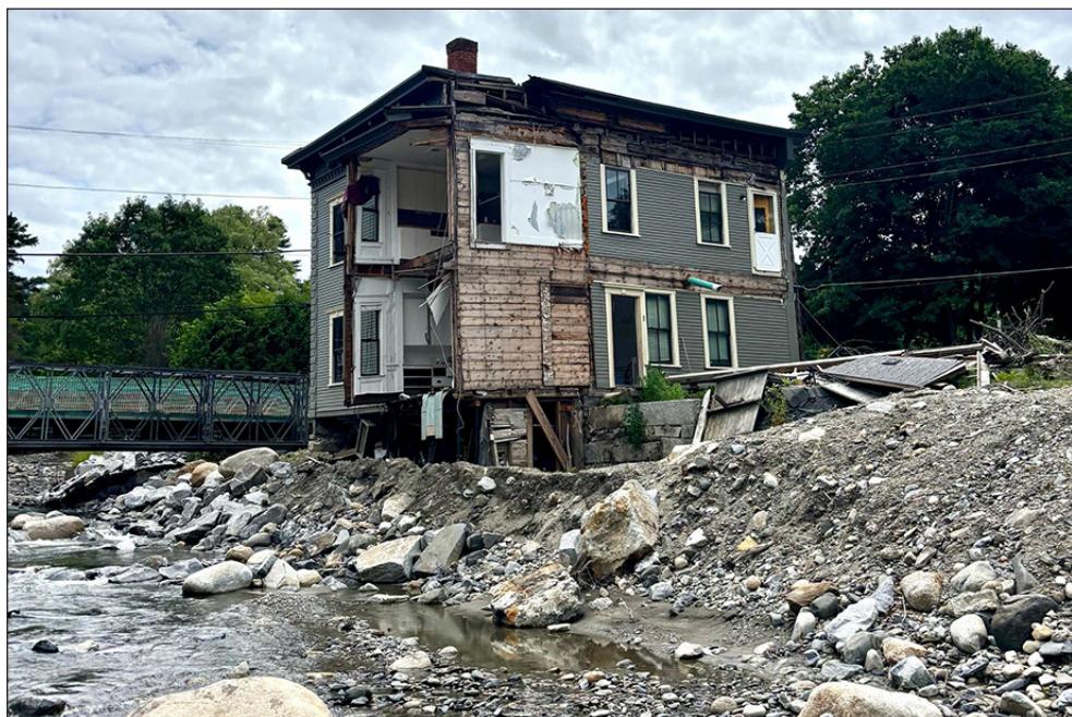
The Heartbreak Hotel in Plainfield was destroyed when Hurricane Beryl reached Vermont as a post-tropical storm in July 2024.
