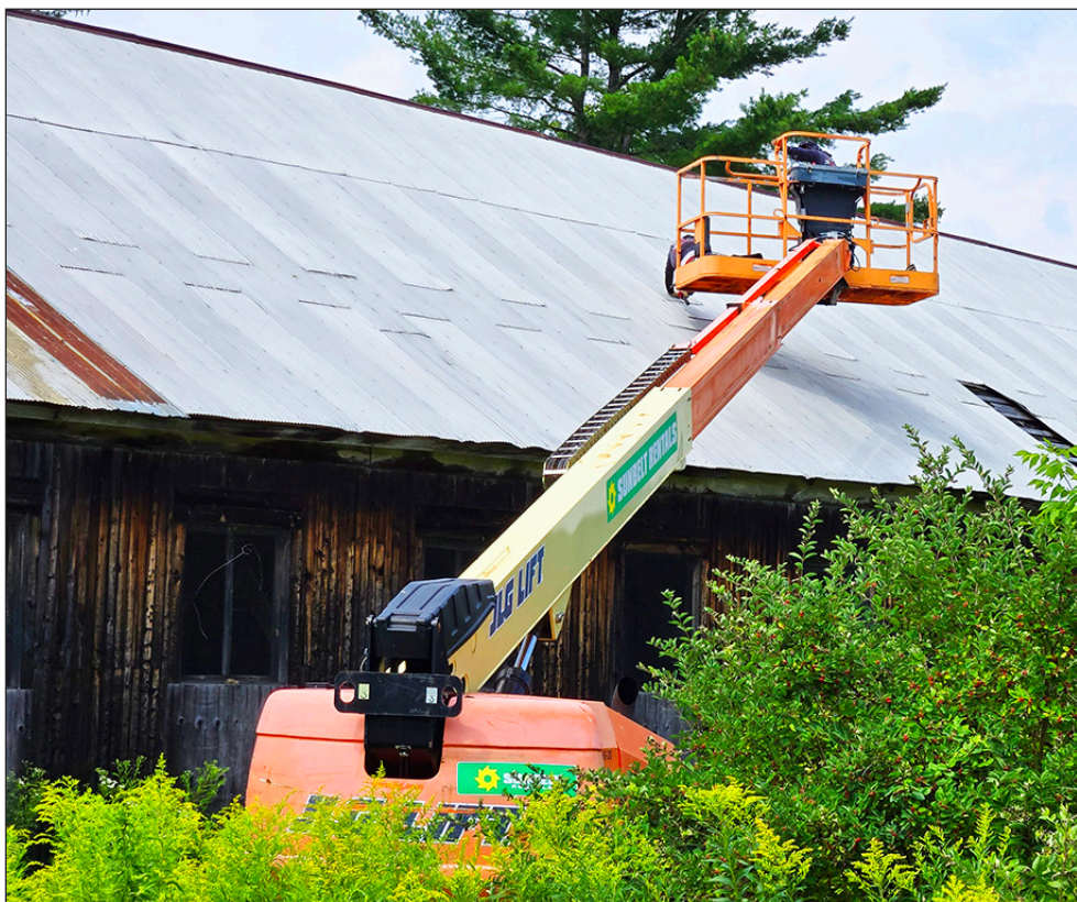
A JR Quality Construction Crew replace missing roofing and fasten loose panels on the Atkins Field granite shed in Hardwick owned by the Center for an Agricultural Economy. photo by Paul Fixx
