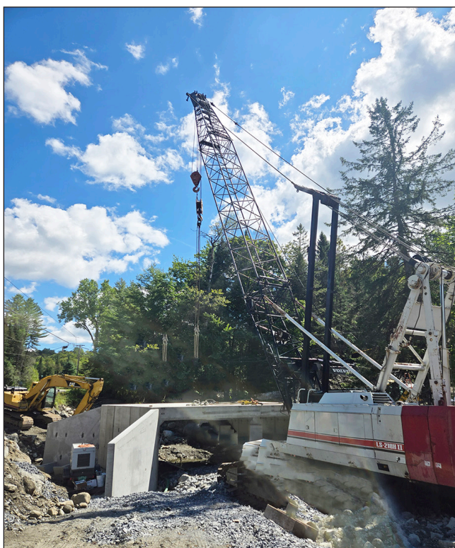
The Orton Road-Richards Road’s new concrete bridge deck and wing walls in place, Sunday, August 31. The bridge in Walden is near the road’s intersection with Stannard Mountain Road and just east of the Lamoille Valley Rail Trail.
