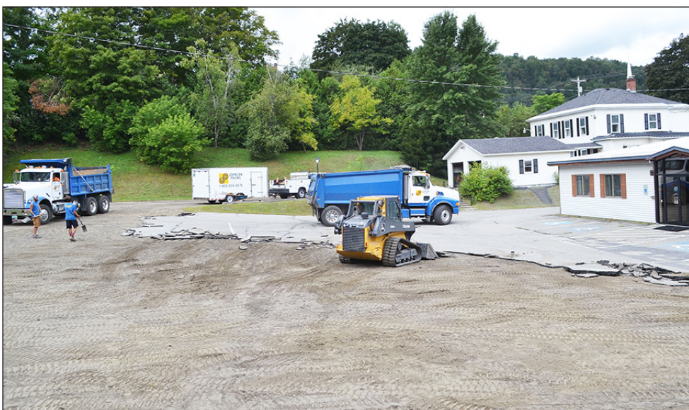
Johnson Paving Company workers of Barre pull up the old pavement at Mary Queen of All Saints Parish St. Norbert Church parking lot, August 20.
