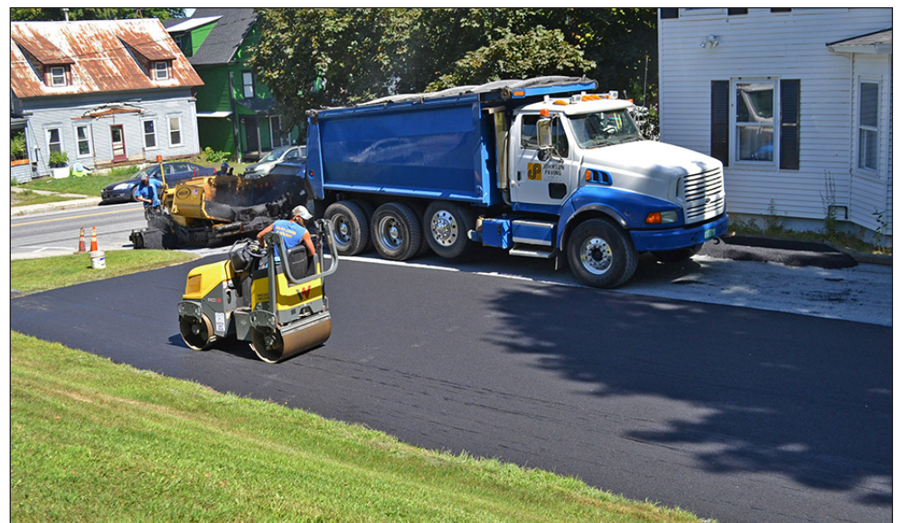
Workers for the Johnson Paving Company put down new asphalt on the Mary Queen of All Saints Parish St. Norbert Church parking lot, August 21 and 22.
