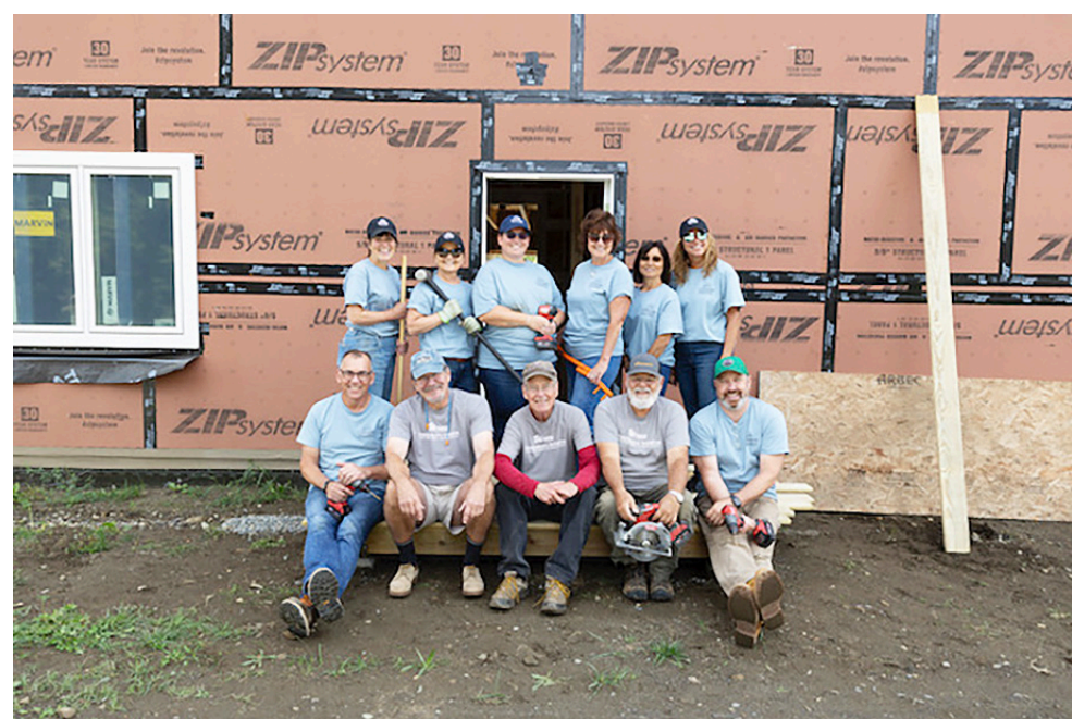
The Central Vermont Habitat for Humanity Greensboro Initiative construction crew in Greensboro Bend, Sept. 5, included area residents and Community National Bank (CNB) executives from Newport, (from left), front row, Chris Caldwell (CNB), Rick Ely, Kent Hansen, Billy Hardy and Justin Bourgeois (CNB), back row from CNB, Tracy Roberts, Louise Bonvechio, Kayla Wright, Regan Howard, Kimico Perry and Kelly Paul. photo by Karen Gowen
