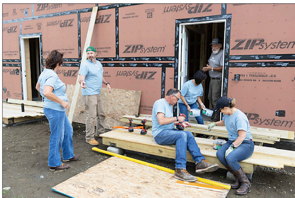
Site Supervisor Billy Hardy (left) oversees Community National Bank executives from Newport working on the Habitat for Humanity duplex home being constructed in Greensboro Bend, Sept. 5. photo by Karen Gowen
