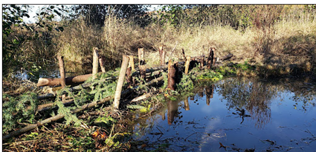
Man-made structures can be used in stream restoration projects to provide some of the benefits of beaver dams, which are porous enough that fish can pass through them. courtesy photo
