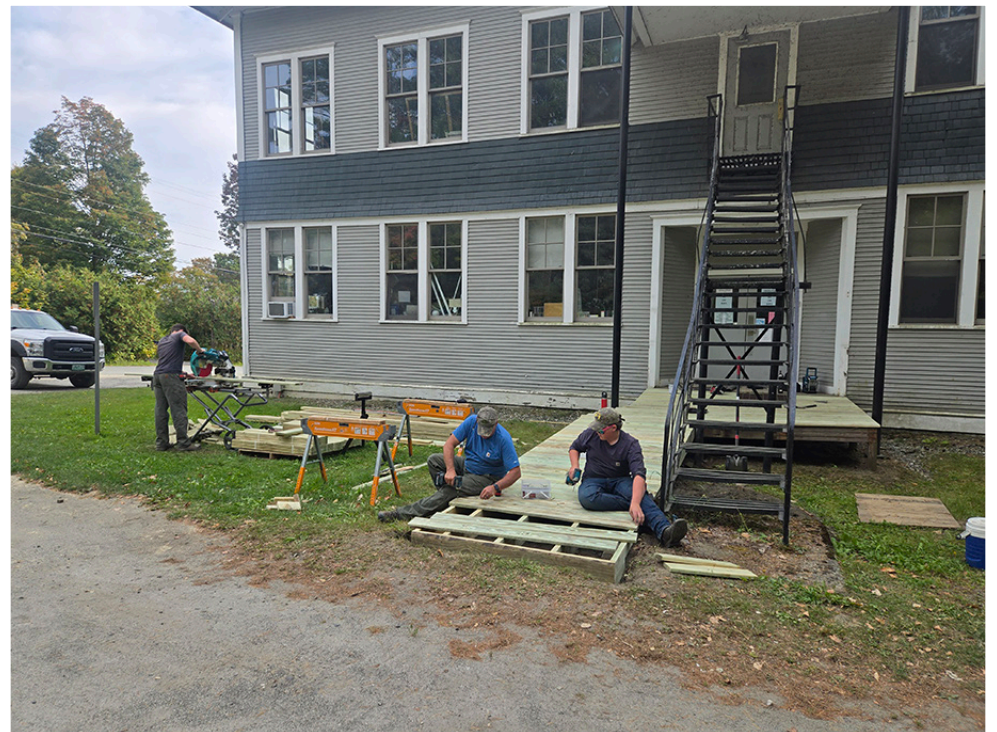
Mike LaPierre (right) works with his sons Lewis (left) and Corbin (center) to replace the ramp at the rear of the Greensboro Town Hall, Monday, Sept. 22. The work was scheduled following the April 29 town vote to abandon a plan to create housing in the building, which would have demolished the deteriorating ramp.
