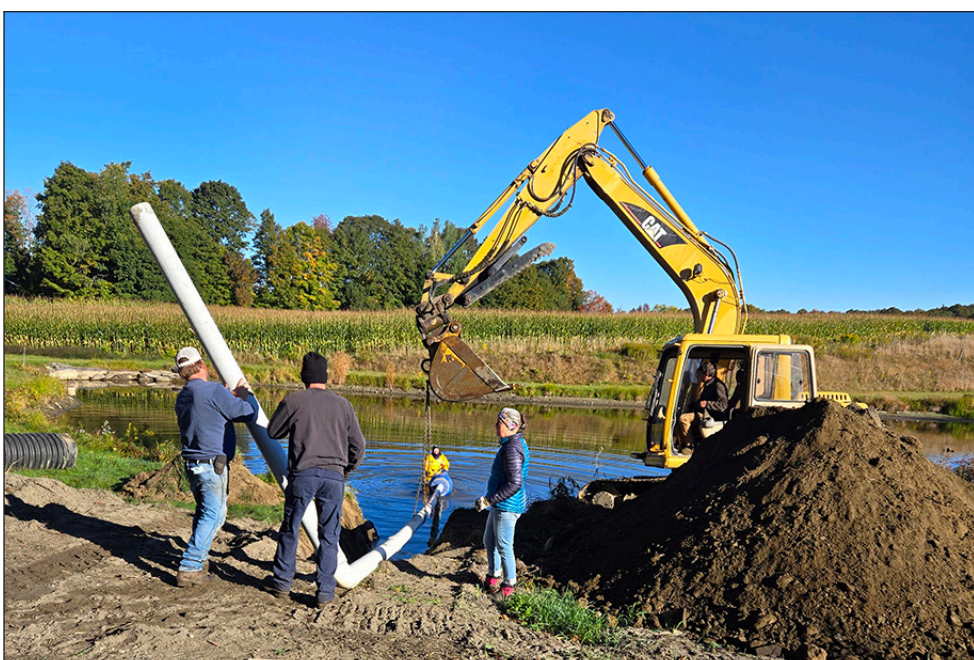
A new fire hydrant is being installed at Brett and Marjorie Urie's pond in East Craftsbury by the Craftsbury Fire Department, by (from left) Asst. Chief Steve Perkins, Captain Robert Hoyt, Lieutenant Andrew Marckres in the pond with the yellow suit, Secretary/Treasurer Thomasina Jacobs and Chief Jeremiah McCann in the excavator, Saturday, Sept. 20. The new hydrant replaces one closer to Greensboro on the same road, that was made unusable when the pool it pulled water from was filled in by 2023 and 2024 flooding.
