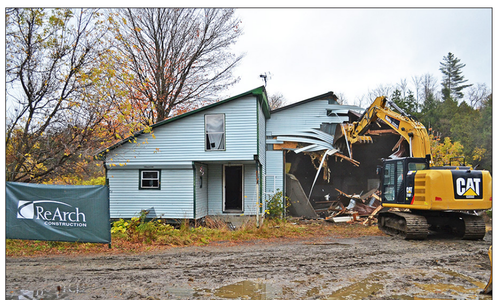
An excavator operated by Mark St. Pierre of Hammond Grinding and Recycling begins the October 8 demolition of the former home of James and Jada Anair on Sawmill Lane in Hardwick. The contents and debris are to be hauled off for proper disposal and recycling. Safety protocols ensured that asbestos and other hazardous materials were handled separately. The project was carried out through FEMA’s Hazard Mitigation Grant Program.
