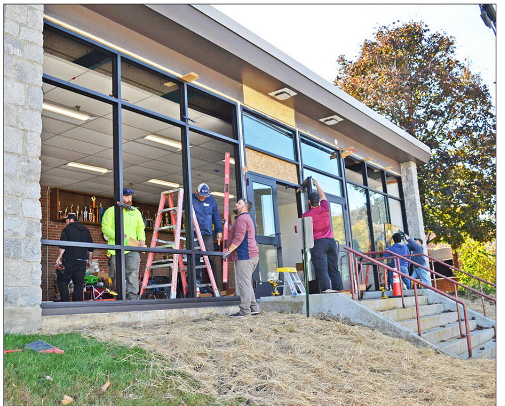
The crew for Burlington Glass were hard at work, October 10, installing frames and windows in the Hardwick Elementary school gym lobby entrance. After four months of abatement and reconstruction work by Energy Efficient Investments, classrooms have reopened with just a few minor details left to be completed.
