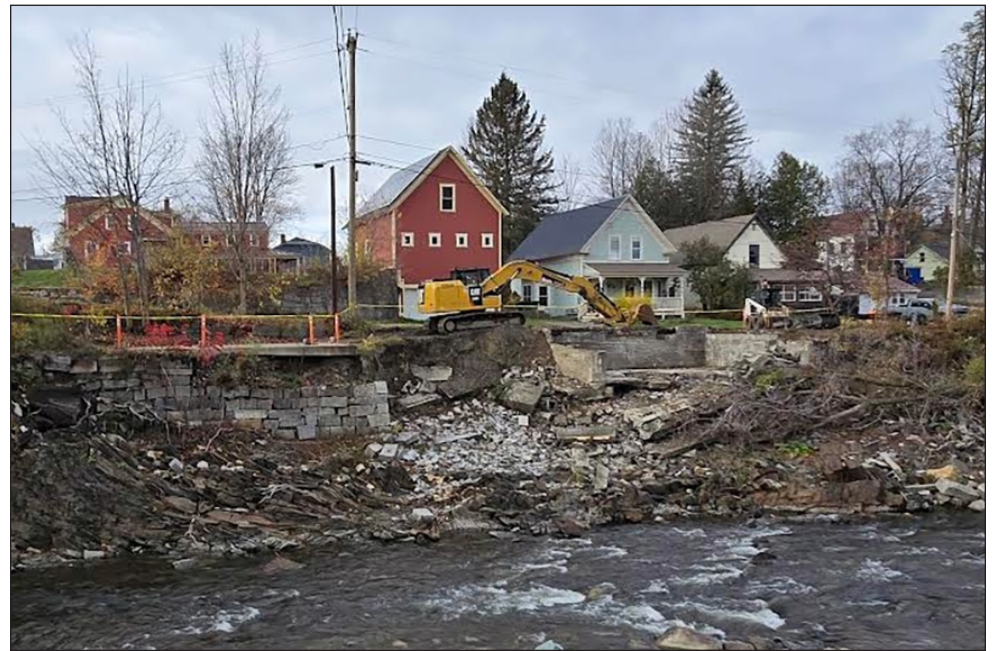
The view across the Lamoille River from behind the Hardwick Inn on South Main St., Wednesday, Oct. 22, no longer includes the home and garage at 41 Brush St. in Hardwick, which is being removed by demolition contractor F.C. Hammond & Son of Orange, N.H., specialists in construction waste management. photo by Paul Fixx
