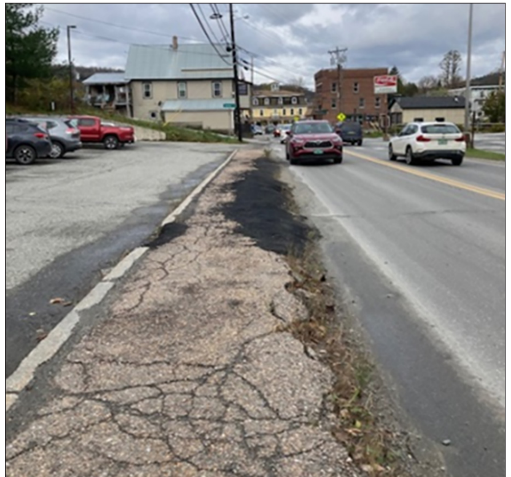
The Mill Street sidewalk in Hardwick, with uneven footing and limited accessibility, next to the public parking area across from the Buffalo Mountain Market, is one of several locations identified as needing safety improvements. photo by Shari Cornish
