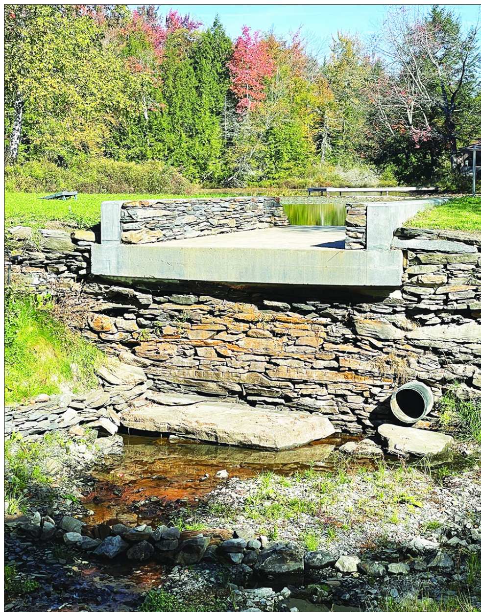
The newly reconstructed Curtis Pond dam in Maple Corner on October 5, 2025. photo by Mason Singer
