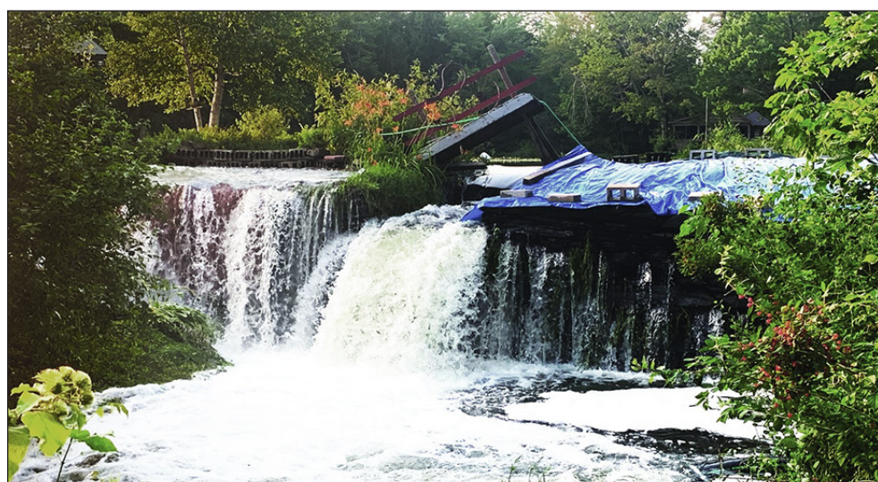
The historic Curtis Pond dam in Maple Corner overwhelmed and near washing out on July 11, 2013. photo by Betty Copeland
