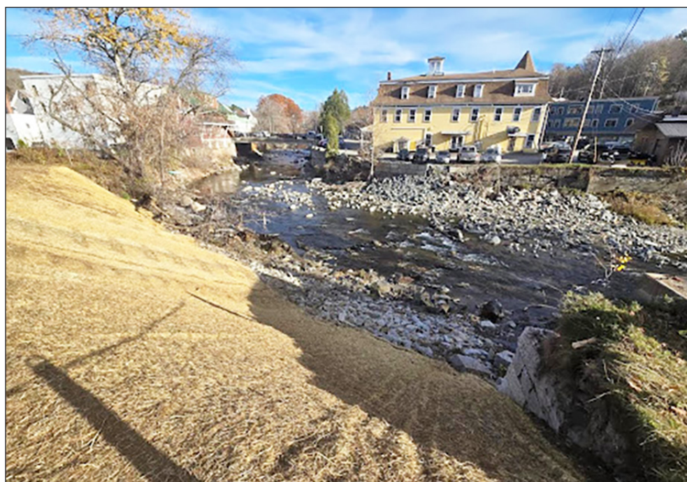
FEMA funded demolition of 41 Brush Street is complete in this view of the Main Street bridge to the left of the Hardwick Inn, showing vulnerability of the river bank to future Lamoille River high water events as the river enters Hardwick's downtown. photo by Paul Fixx
