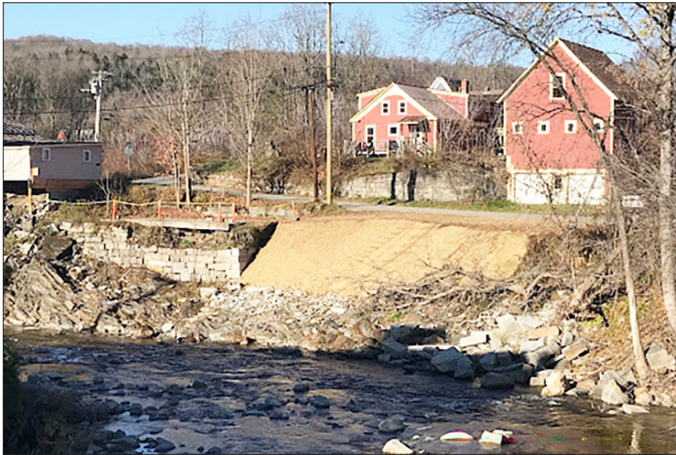
Following a federal buyout that transferred ownership of 41 Brush Street to the Town of Hardwick, the home and garage that once stood there has been removed, while the stone retaining wall continues to hold the Lamoille River's bank, supporting a concrete slab left in place. photo by Kristen Leahy
