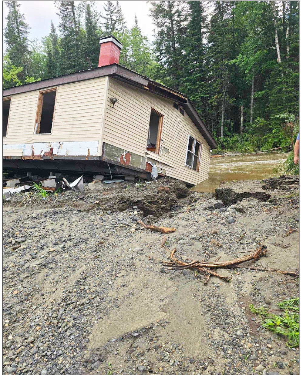
The house at 387 Carey Road, purchased in a buyout after repeated flood damage and 2023 flooding, is seen here in mid-demolition after the 2024 flood hit. photo by Kristen Leahy
