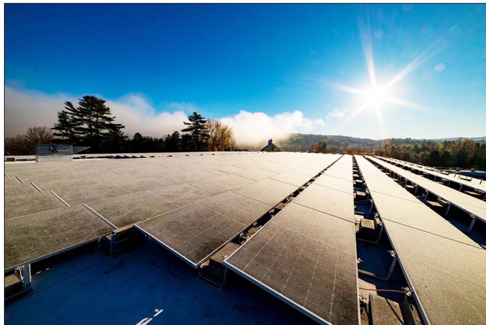
The Center for an Agricultural Economy's solar array on the Hardwick Food Hub rooftop was completed in October. courtesy photo
