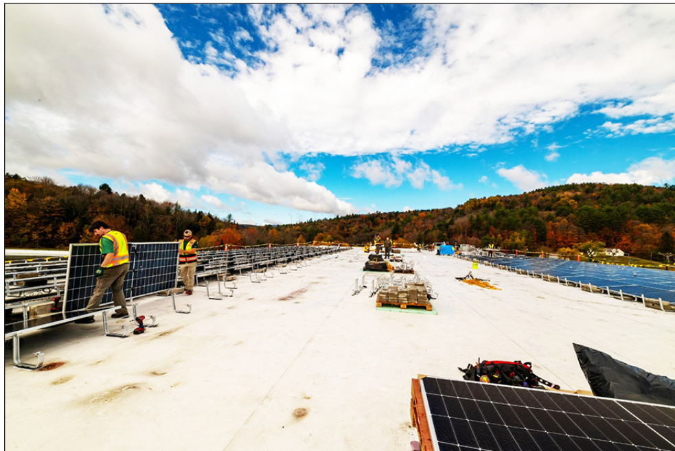
A solar array under construction on the roof of the Center for an Agricultural Economy's Hardwick Food Hub earlier this year. courtesy photo
