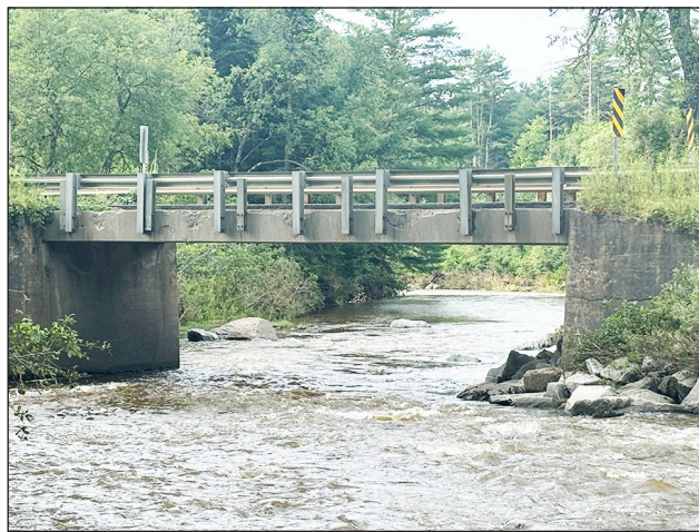
The current Gulf Road Bridge to be replaced over the Wild Branch in Wolcott. courtesy Lamoille County Planning Commission
