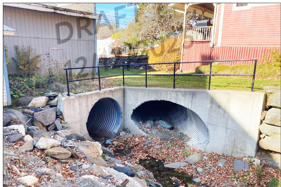
A photo from the December 12 draft, “Cabot garage relocation site assessment,” shows culverts at the rear of the current Cabot Garage, which is planned for removal with a contract expected to be signed soon for flood mitigation work by Dubois & King.
