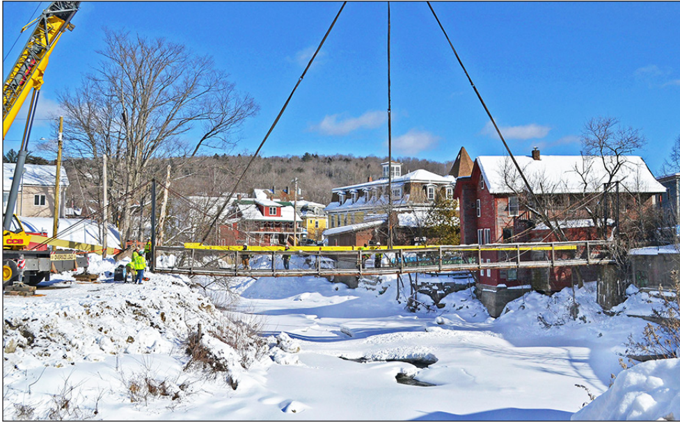
CCS Constructors of Morrisville prepare the pedestrian bridge for its February 5 removal in Hardwick Thursday. photo by Vanessa Fournier
