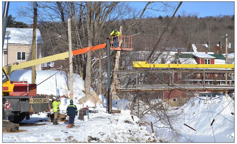
A worker from CCS Constructors removes cables from the 18 foot steel suspension tower connected to Hardwick's historical pedestrian foot bridge. photo by Vanessa Fournier
