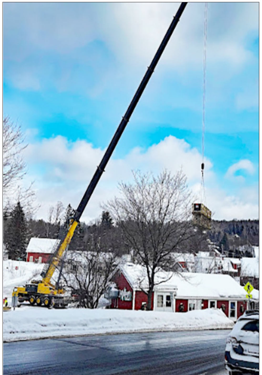
A CCS crane lifts a temporary bridge from the Main Street side of the Lamoille River in Hardwick village to the parking lot beside the Daniels Building, February 4. The work began the long-anticipated project to replace Hardwick's swinging bridge. Work came to halt following removal of the old bridge last week until March when it's anticipated replacement of the South Main Street retaining wall will begin work leading to replacement of the pedestrian bridge.
