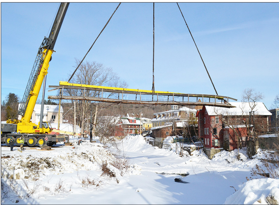
A CCS crane lifts the circa 1915 102 foot swinging bridge February 5 in Hardwick which connected Main Street to Brush Street for over 100 years. The foot bridge was closed in August 2020 due to a failed suspension system. photo by Vanessa Fournier
