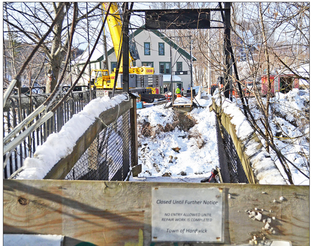
Hardwick's swinging foot bridge was removed, February 5, by CCS Constructors of Morrisville. Rebuilding the Main Street retaining wall will begin in early March and after that is completed, a new pedestrian bridge will be installed. The project is scheduled to be finished by mid-November. photo by Vanessa Fournier
