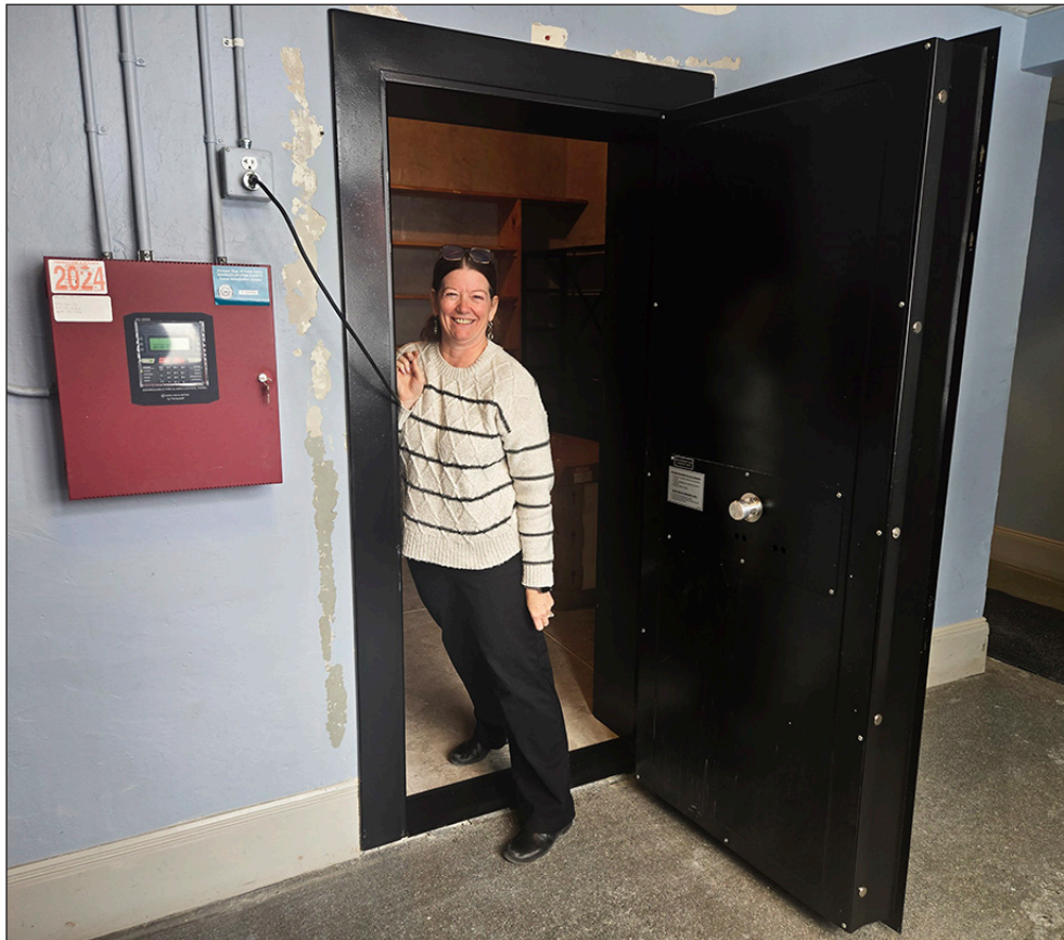
Hardwick Town Clerk Tonia Chase stands in the doorway of the vault on the Memorial Building's first floor, where a new, wider door has just been installed, Thursday, February 11. The space was once filled with boxes piled on the floor that made use of the space difficult, she said. photo by Paul Fixx
