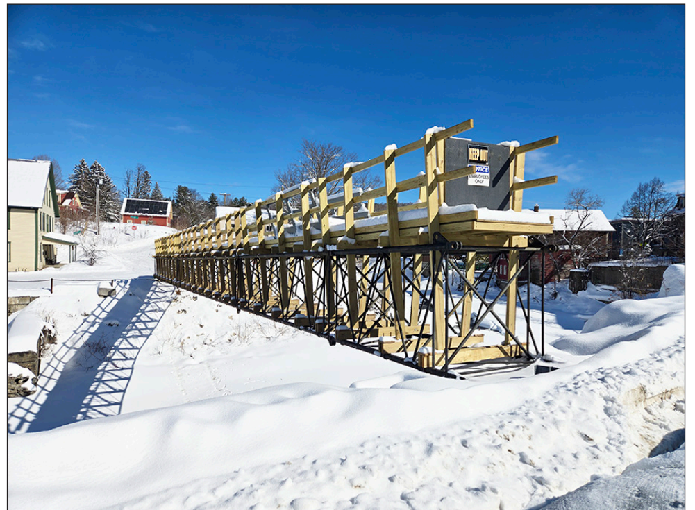
A temporary bridge that workers will use during reconstruction of a retaining wall along Main Street between the Village Restaurant and the former swinging bridge, is placed across the river awaiting its spring installation.
