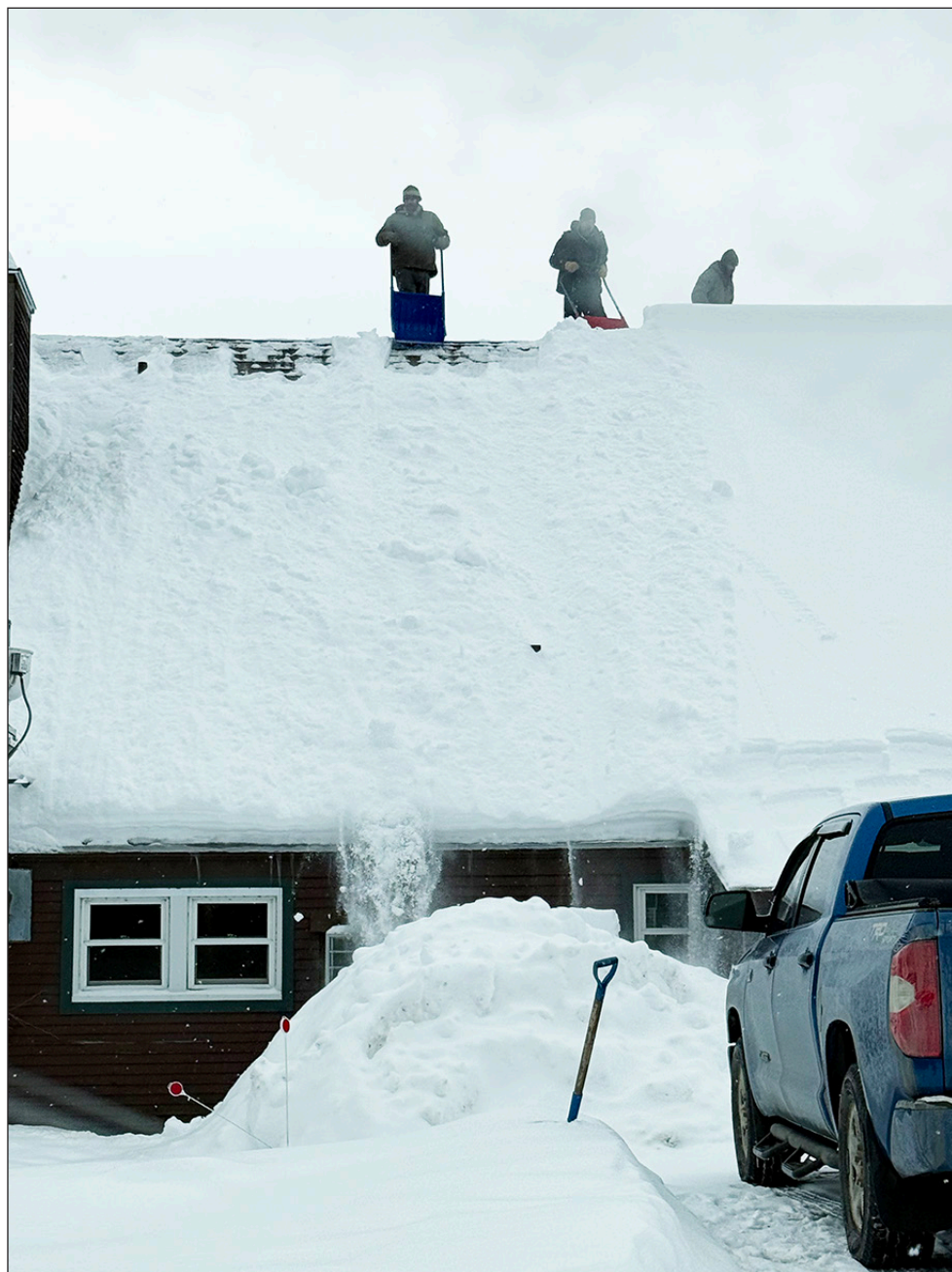
A crew shovels snow from the roof of the Greensboro Nursing Home last Wednesday.
