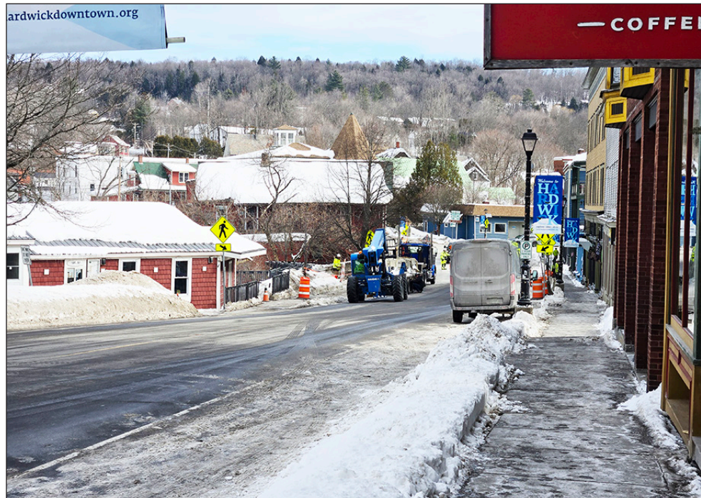
Construction crews begin preparing for work on the retaining wall and pedestrian bridge beside Hardwick's South Main Street that will reduce the area to a single lane into early summer. Three traffic lights now control vehicular movement through the area. photo by Paul Fixx
