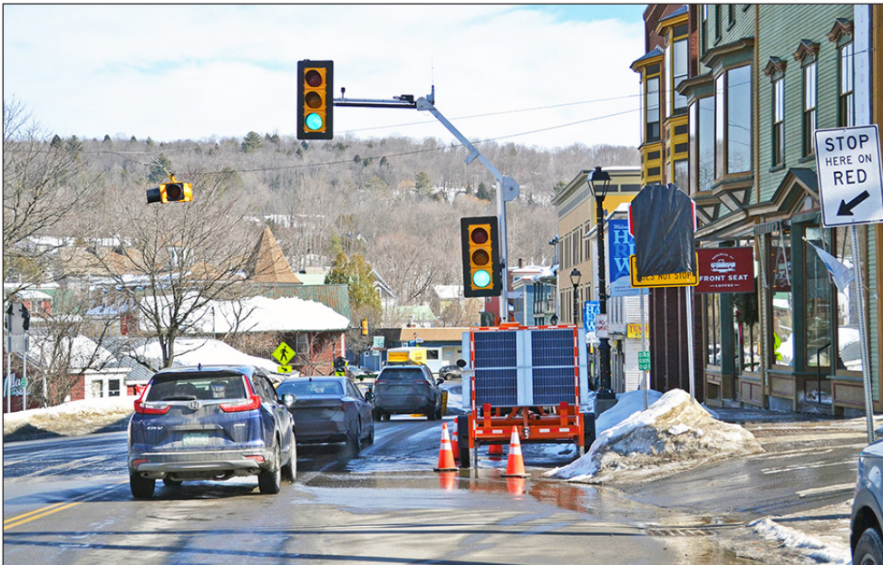
Work by CCS Constructors on the South Main Street retaining wall and pedestrian bridge project began February 27 in Hardwick. Traffic will be one lane with alternating traffic lights on South Main, Mill and Wolcott Streets (Vt. Routes 14 and 15), with another light directing traffic exiting the Village Restaurant parking lot onto Wolcott St. photo by Vanessa Fournier
