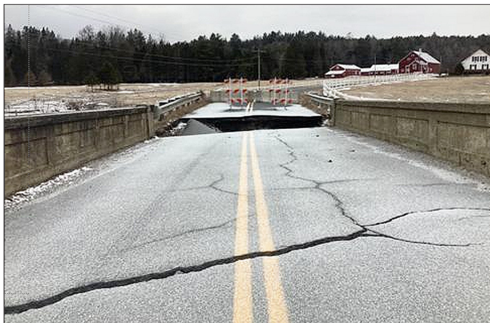
East Hardwick’s Bridge 31 is impassable following July 2023 flooding that washed out the eastern approach and was determined to be structurally unstable. photo courtesy Town of Hardwick
