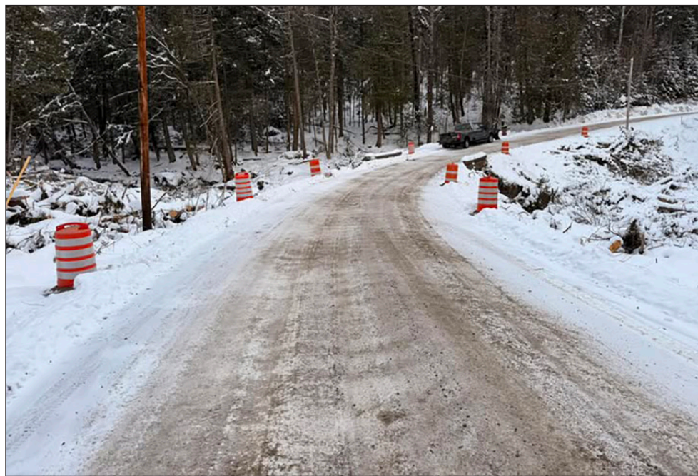
Clearing along Lovely Road in Cabot has been done in preparation for a FEMA bridge replacement scheduled to begin after July 1 this year.
