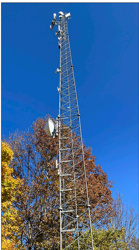
The new WGDR antenna will be located on this tower, 1,000 feet higher and on a ridge, allowing for much wider distribution of the broadcast signal.
