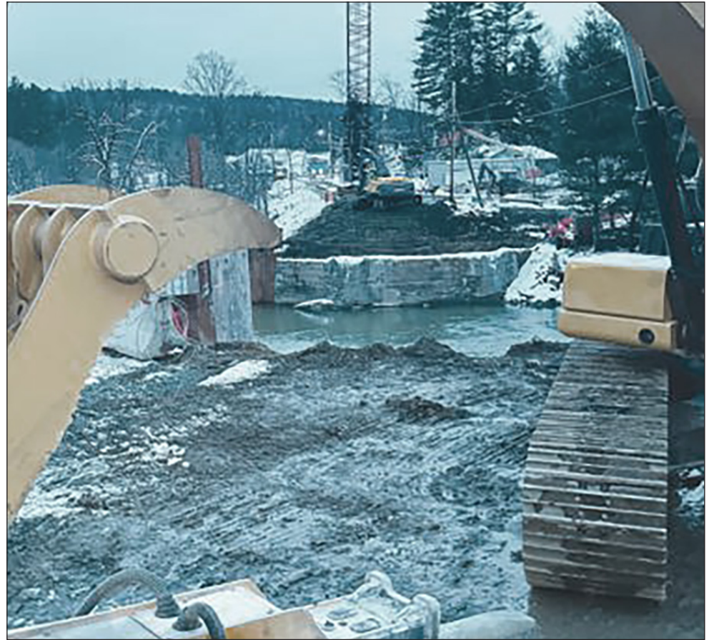
You can't get there from here: Drivers will have to take the long way around the Lamoille River to access School Street in Wolcott for the next half year, as workers replace a nearly-century-old steel truss bridge.
