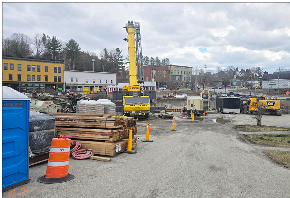
Downtown Hardwick serves as a backdrop for construction equipment being used on reconstruction of the South Main Street wall and pedestrian bridge, Saturday. photo by Paul Fixx
