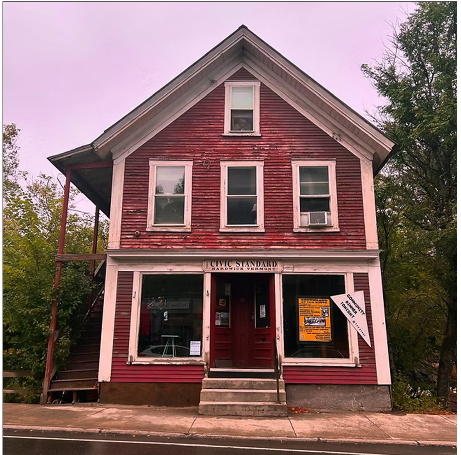
The home of the Civic Standard from May 2022 to late 2025, at 42 S. Main St. in Hardwick now stands empty, with only a FEMA buyout, demolition and becoming green space as an option for its future. It was the home of The Hardwick Gazette for more than 100 years before The Gazette moved to Greensboro in 2021.
