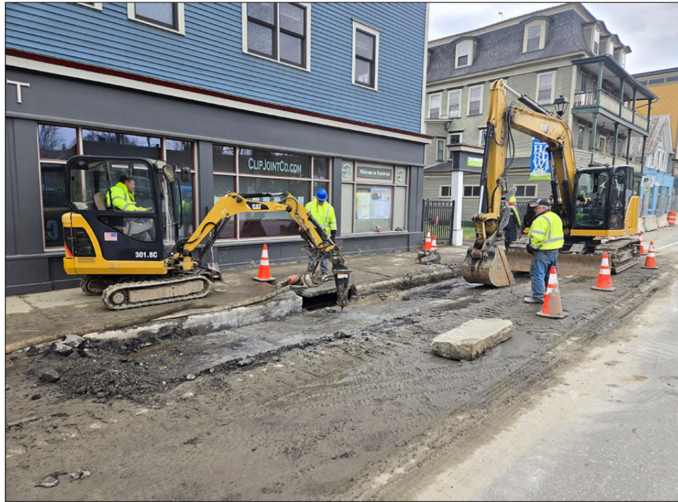
Members of the Hardwick Road Crew work to uncover a leaking water main on S. Main St. in front of the Clip Joint, Wednesday, April 22 shortly after noon. The break was repaired by that evening and a boil water notice was lifted Saturday morning. photo by Paul Fixx
