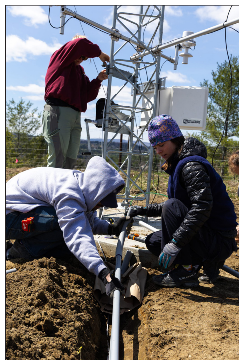
UVM Water Resources Institute interns, Maeve Dewey and Liam Muskin, install a soil sensor and rain gauge on the tower of an extreme weather monitoring station, with Samantha Koehler, Senior Meteorological Technician, adjusting the tower's alignment, near the Vermont State University campus in Lyndonville.
