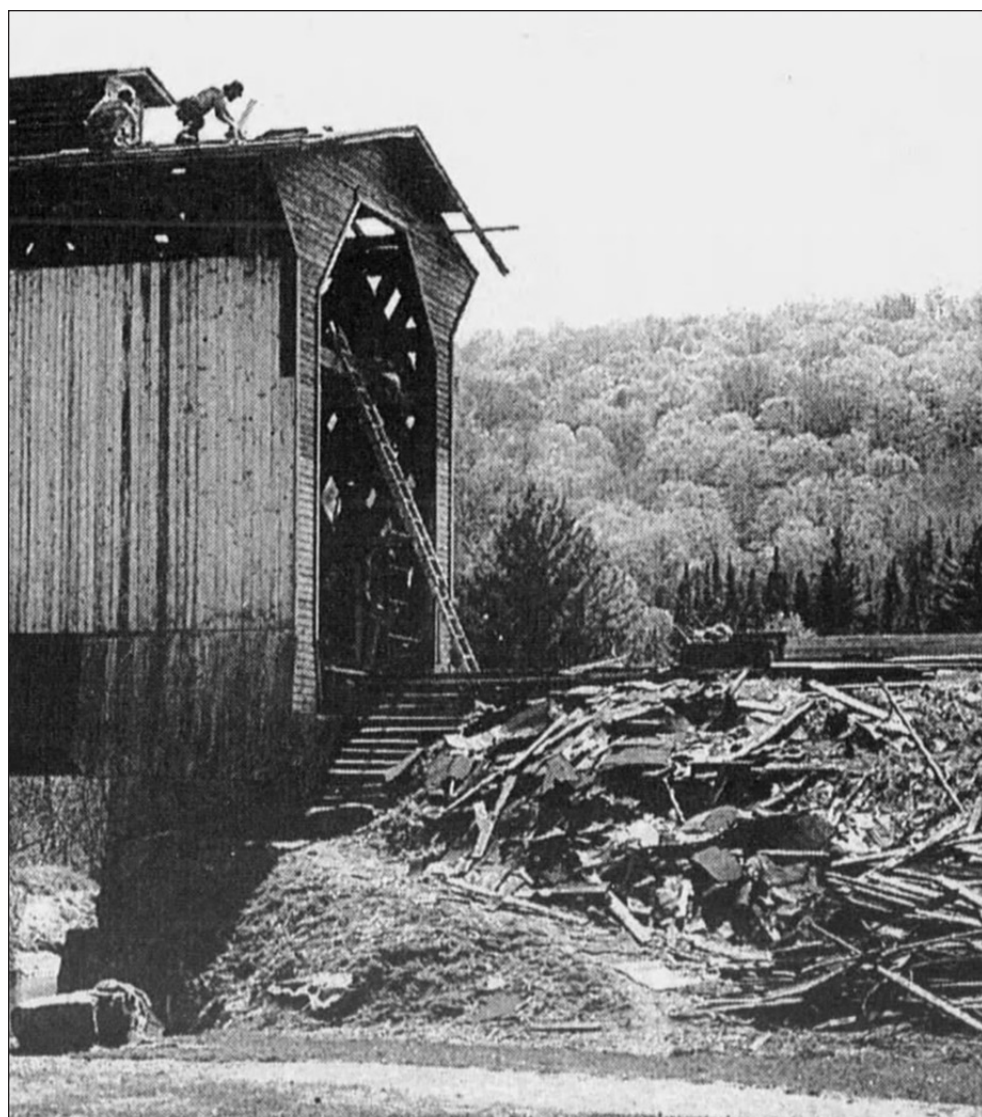
Workers repaired the roof of The Fisher Bridge last week, bringing to a close a 10 year project to restore the structure. Once the last used railroad covered bridge in the country, the state secretary of transportation is expected to announce this week that the rail corridor will be turned into a trail. (photo by Jo Gilder), The Hardwick Gazette, May 16, 2001
