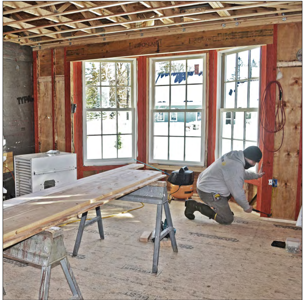
photo by Vanessa Fournier Kingdom Construction Inc. foreman Dwayne Bowen works last week on the 14 x 24-foot Leesa Fine Room addition to the Craftsbury Public Library.
